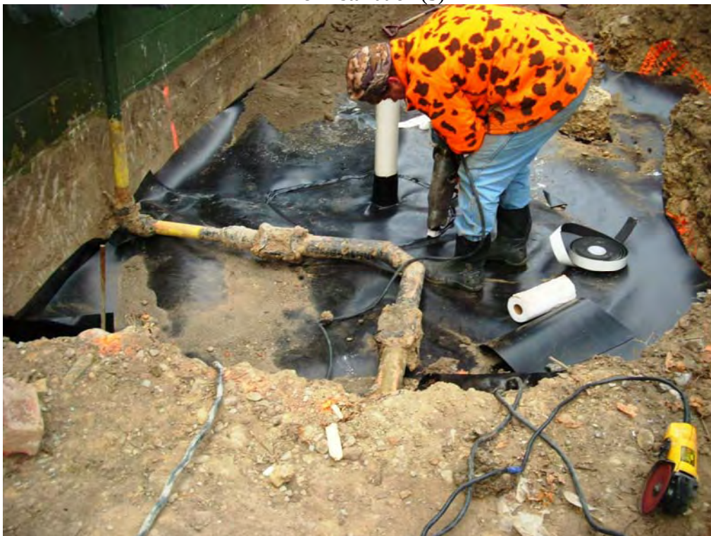
Welding seam around vapor well
