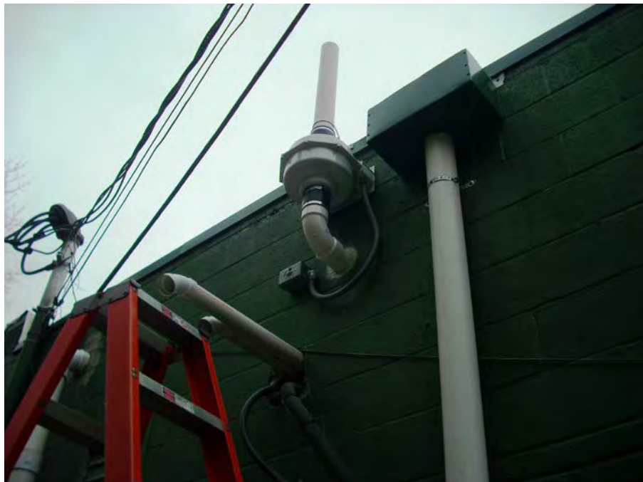
Installed Fan Exterior
