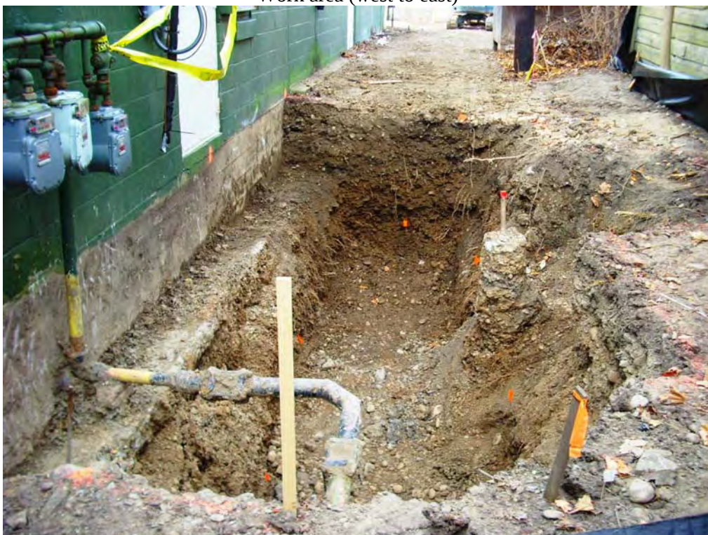
Exposed Gas line and view of west end of excavation
