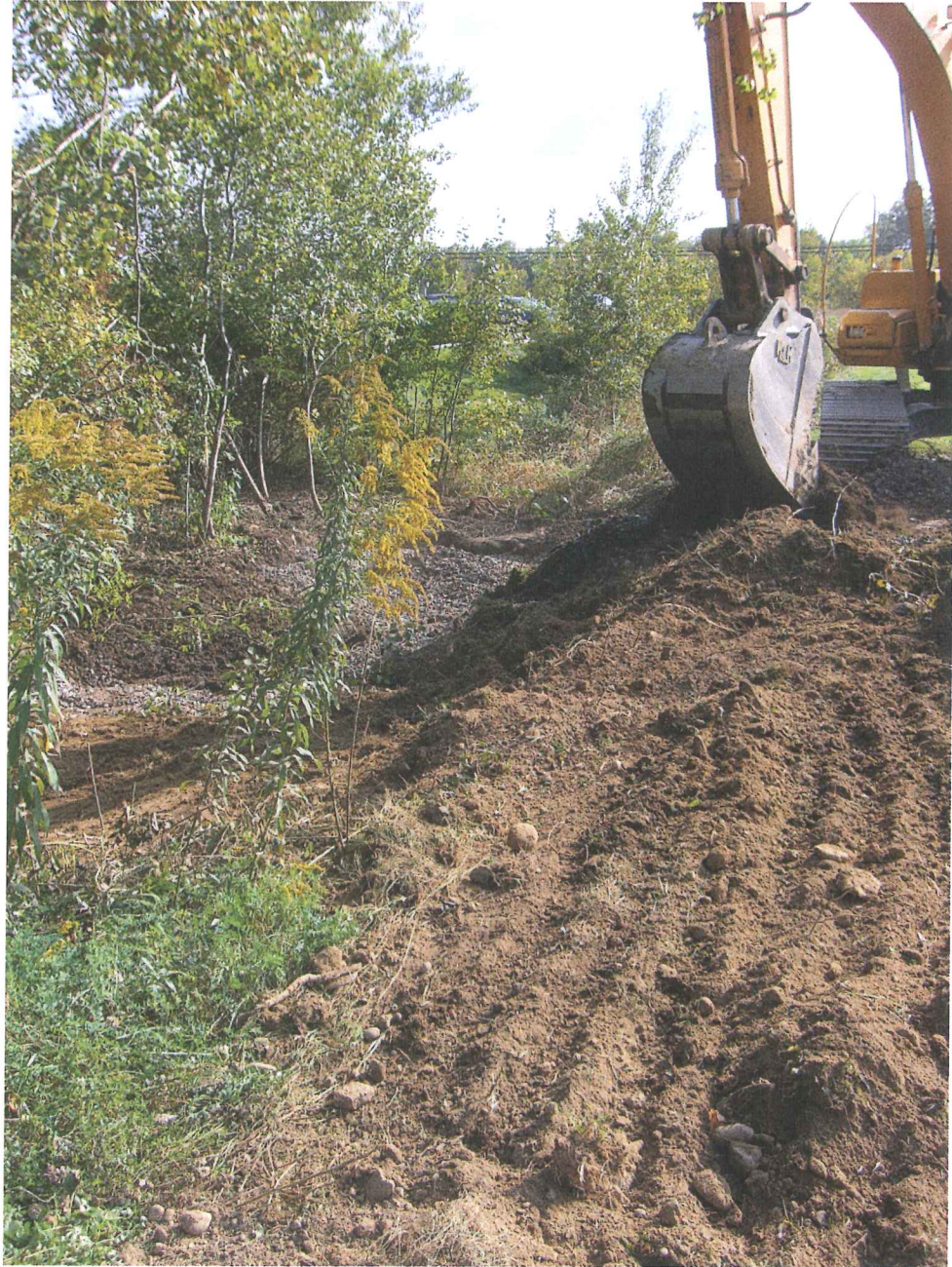
Picture 4 – Completion of drainage ditch backfill using onsite soils scraped from berm between ditch and pavement.
