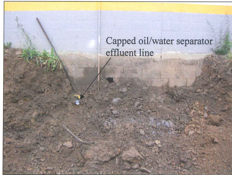
Picture 3 – UST excavation at building wall showing capped oil/water separator effluent line.
