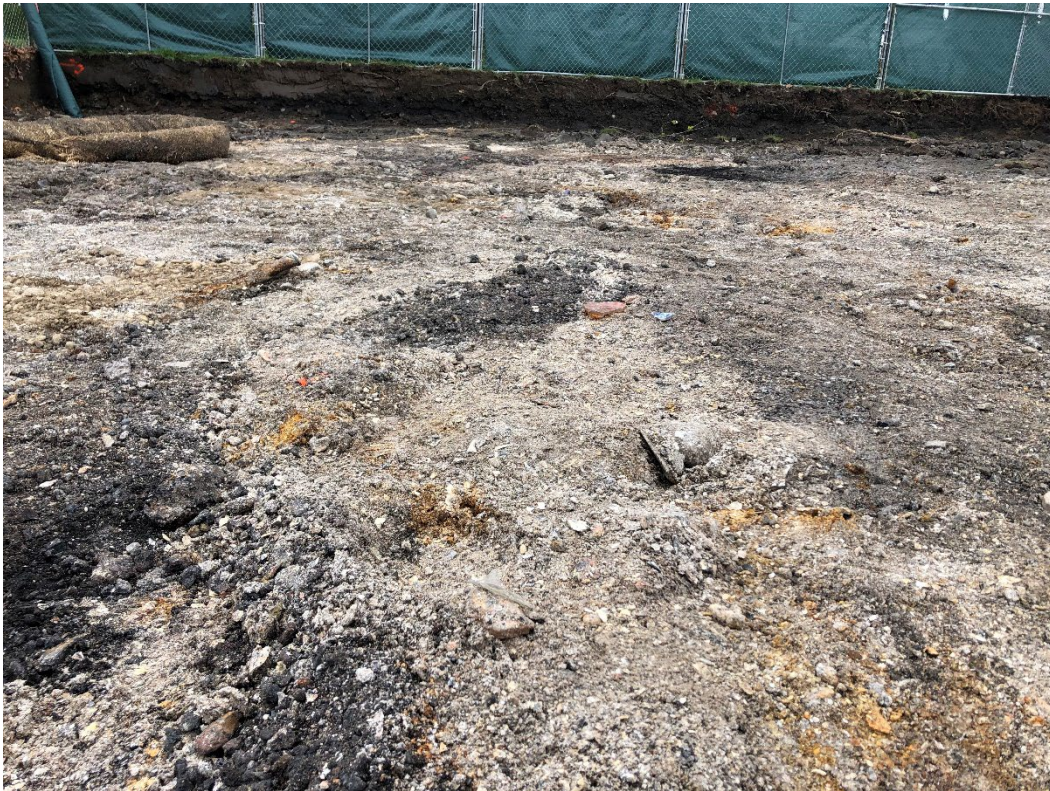
Picture 3: Excavation heavily impacted with ABG.
