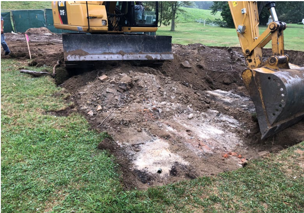
Picture 2: Excavation heavily impacted with ABG.
