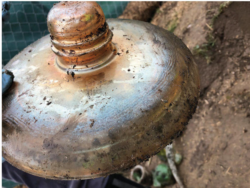
Picture 21: Opalescent insulator with approximately 1-ft diameter.
