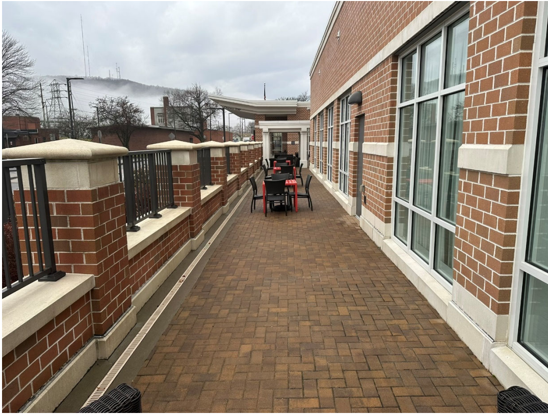
Photograph 5: Patio and stamped concrete cover system in the southeast corner of the building along Riverside Drive (looking west).
