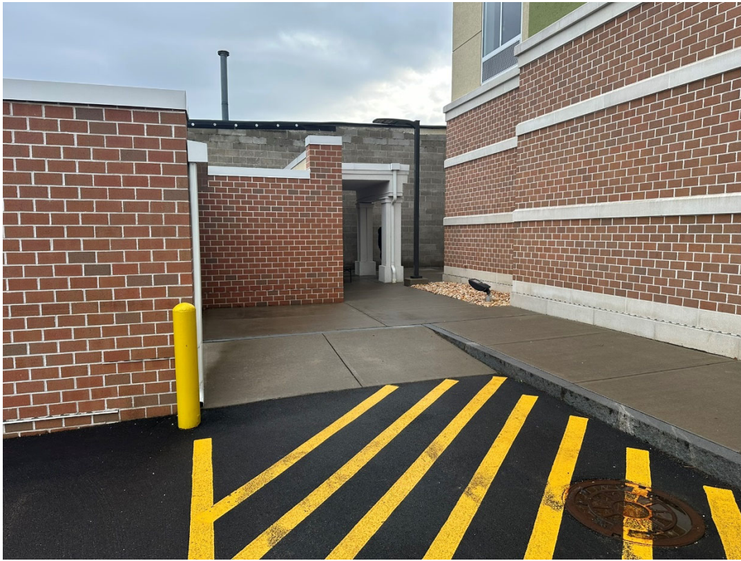
Photograph 11: Concrete sidewalks and back side of exterior storage areas along the northeast corner of the building (looking east).
