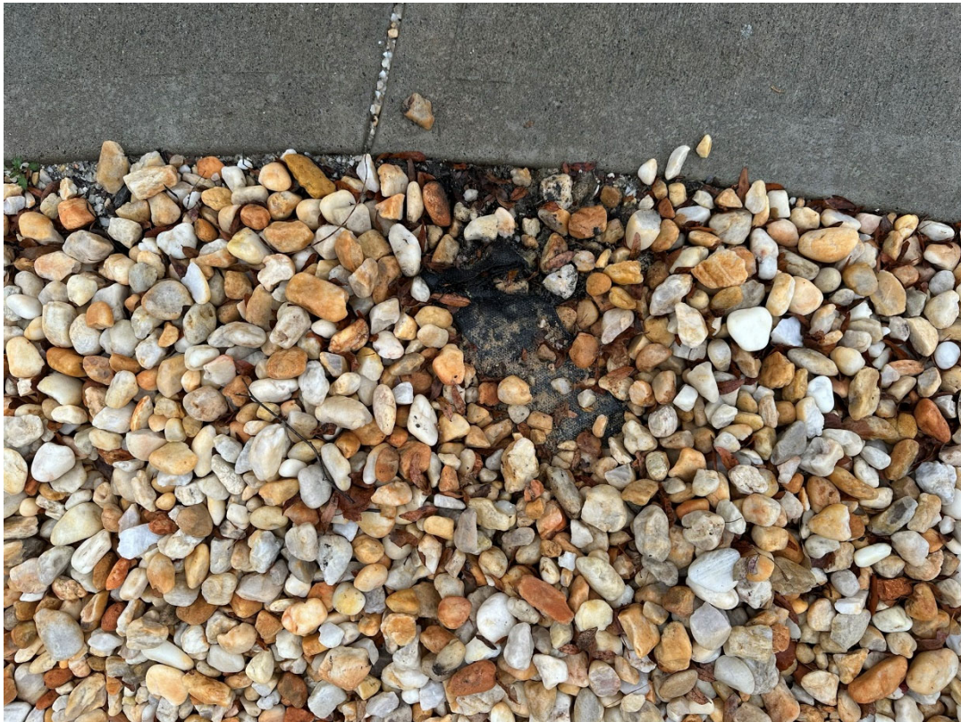
Photograph 10: Black landscape bed fabric beneath riverstone in the northwest corner of the building was left in place after removing mulch in August 2024.
