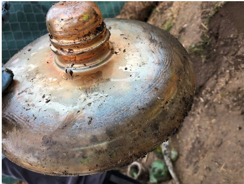
Picture 21: Opalescent insulator with approximately 1-ft diameter.
