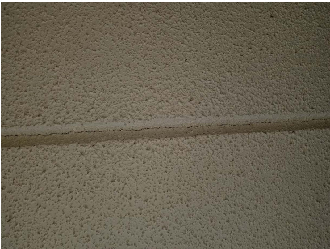
Photograph No. 4 – Photo of hotel room ceiling showing crack in joint between panels.
