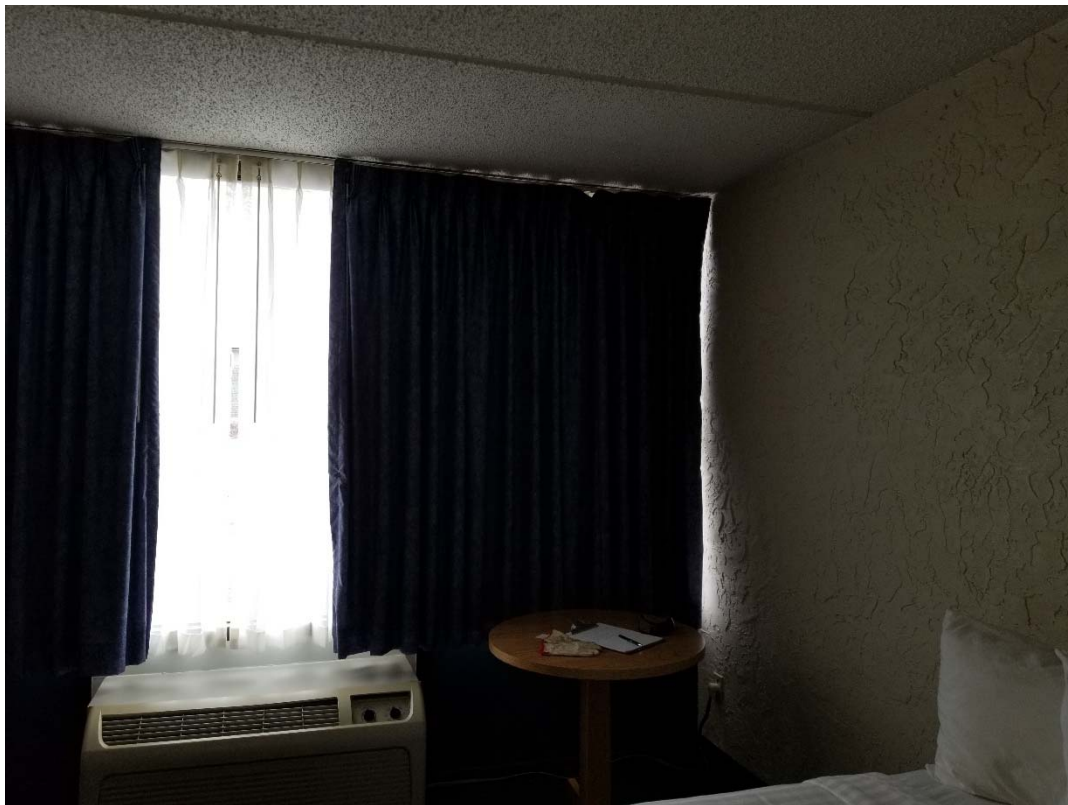
Photograph No. 2 – General view of hotel room's exterior wall (windows and metal paneling) and interior sidewall (stucco finish).
