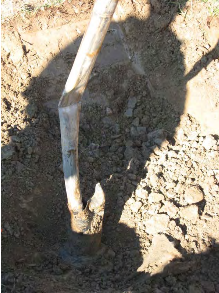
10/17/12: Damaged Piezometer PZ-3R with protective casing and cover soil removed
