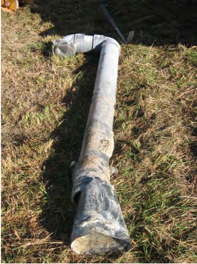
10/17/12: Damaged gas vent V-12
