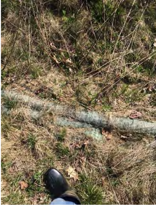
Photo No.5 Exposed geotextile
