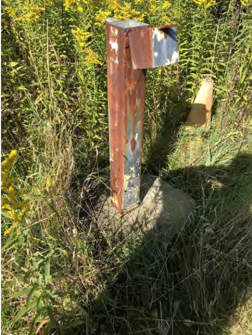
Photo No. 1 MW-1S upheaved
