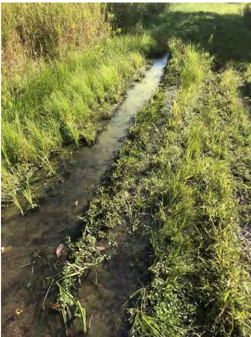
Photo No. 7 Ponding on south edge of Site
