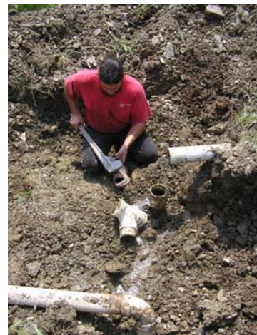
ik BBT1 North Repair 5.J
