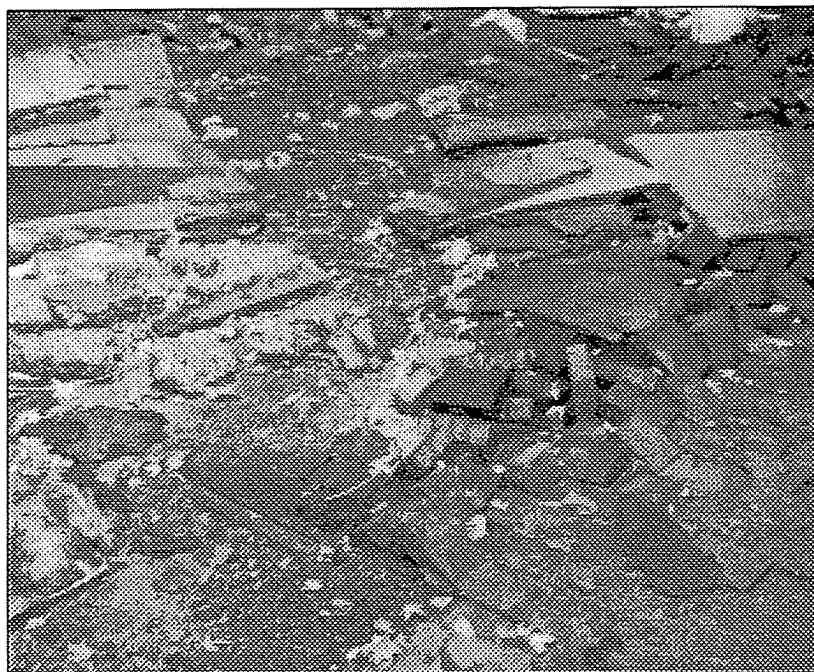
Oil-soaked wood block flooring in East Production Room
