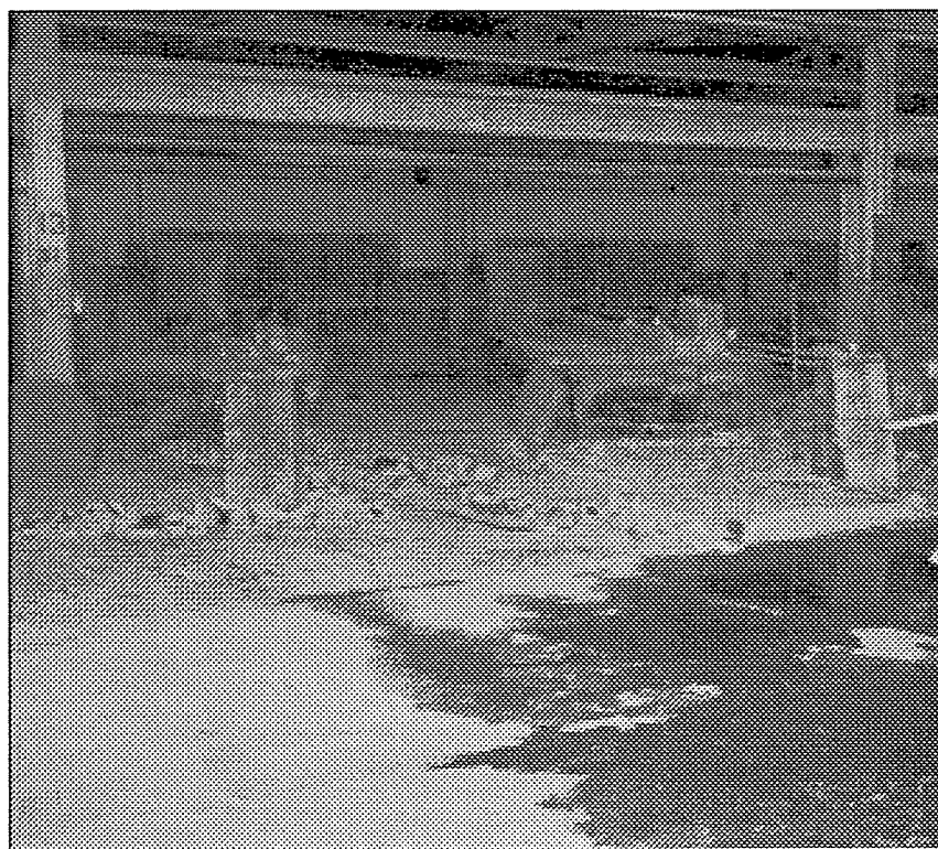
West Production Room, looking south toward Transformer Room
