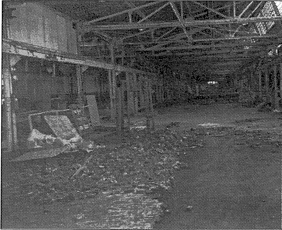
Main aisle of West Production Room, looking west
