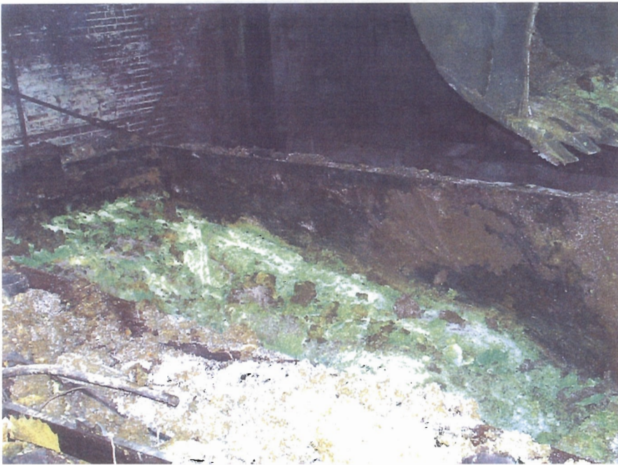
Photo 2. East end of Kolene tank process area after removal of liquefied material
