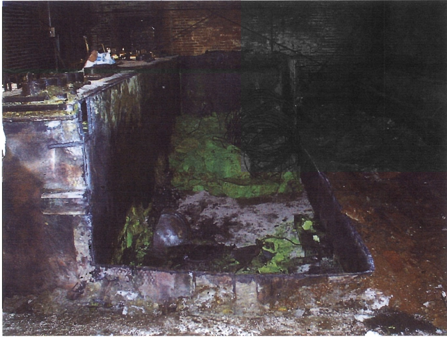
Photo 7. Process portion of tank - looking east after removal of west & south walls
