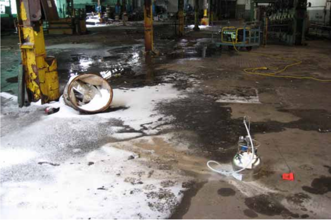
Photo/Frame No.: ALTech Direction of View: East Date/Time: 02/25/08 Subject: Sub-slab sample HW907022-SS05-022508
