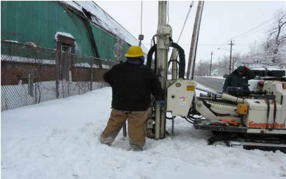
Photo/Frame No.: ALTech Direction of View: West Date/Time: 02/27/08 Subject: Boring location area for B19EA, B19EB, B19WA and B19WA
