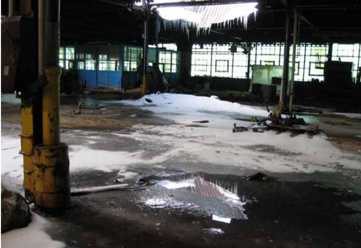
Photo/Frame No.: ALTech Direction of View: Northwest Date/Time: 02/27/08 Subject: Former East Production Area north wall (ceiling starting to collapse)
