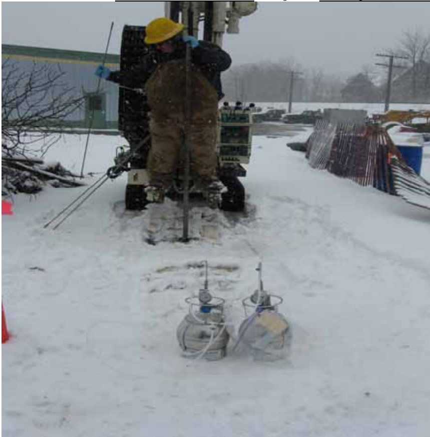
Photo/Frame No.: ALTech Direction of View: East Date/Time: 02/26/08 Subject: Boring location area for V02 (with duplicate sample V06)
