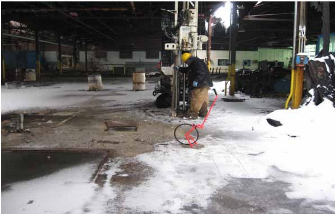
Photo/Frame No.: ALTech Direction of View: West Date/Time: 02/26/08 Subject: Boring location B21W (soil samples) in Former East Production Area. Wheel designates ATSS-NP-21-2 location.
