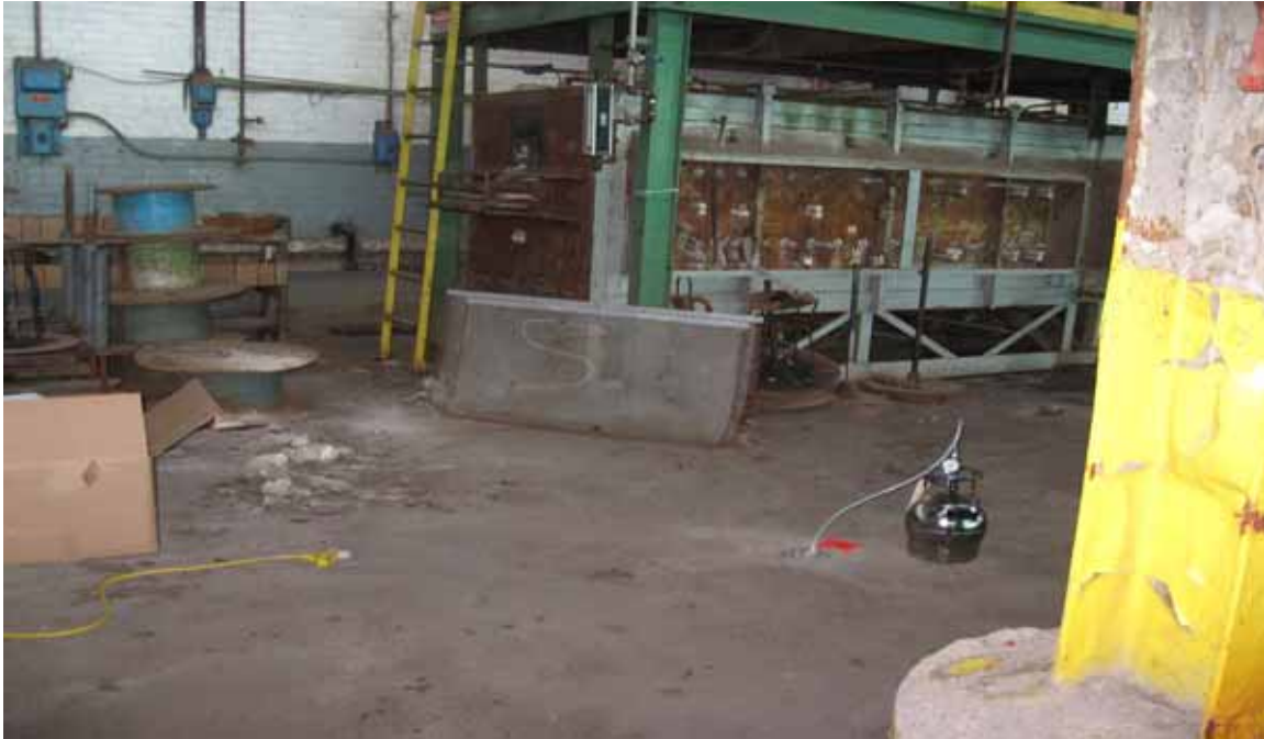
Photo/Frame No.: ALTech Direction of View: Southwest Date/Time: 02/25/08 Subject: Sub-slab sample HW907022-SS01-022508
