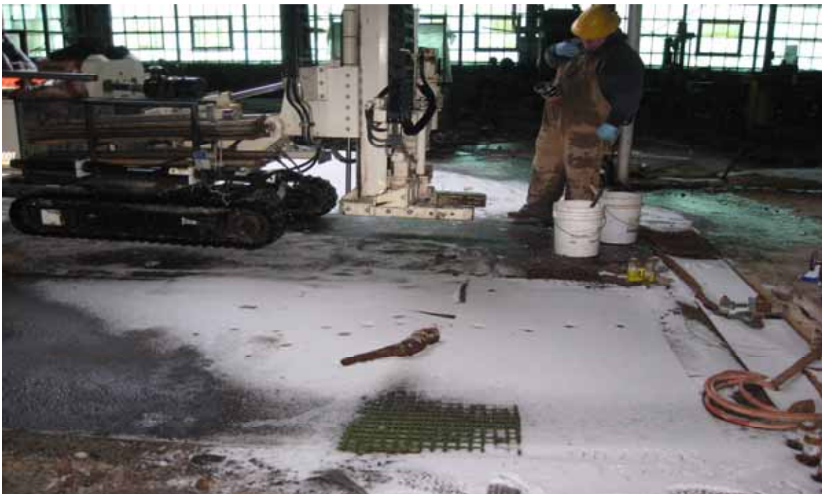
Photo/Frame No.: ALTech Direction of View: North Date/Time: 02/26/08 Subject: Boring location B21E (soil samples) in Former East Production Area
