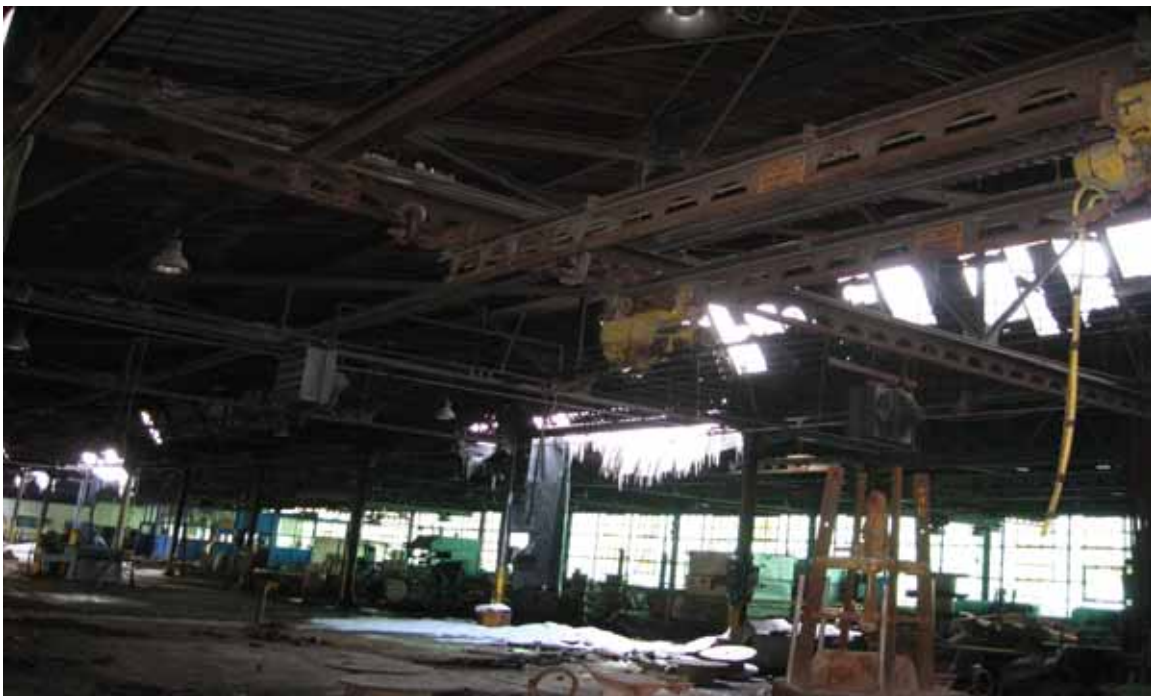
Photo/Frame No.: ALTech Direction of View: Northwest Date/Time: 02/27/08 Subject: Former East Production Area north wall (ceiling starting to collapse)
