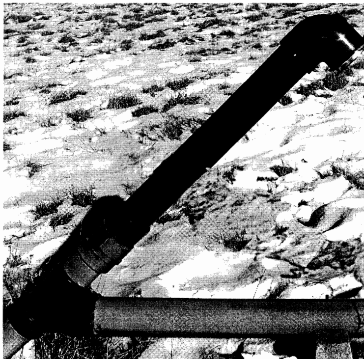
Photo 3 – Installed vent riser with expandable plug inserted.
