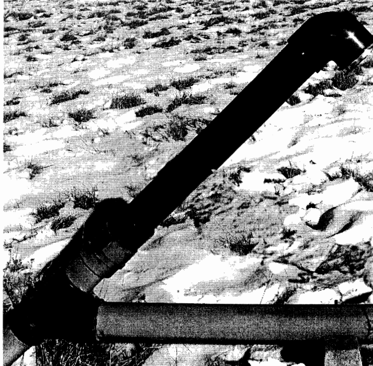
Photo 3 – Installed vent riser with expandable plug inserted.
