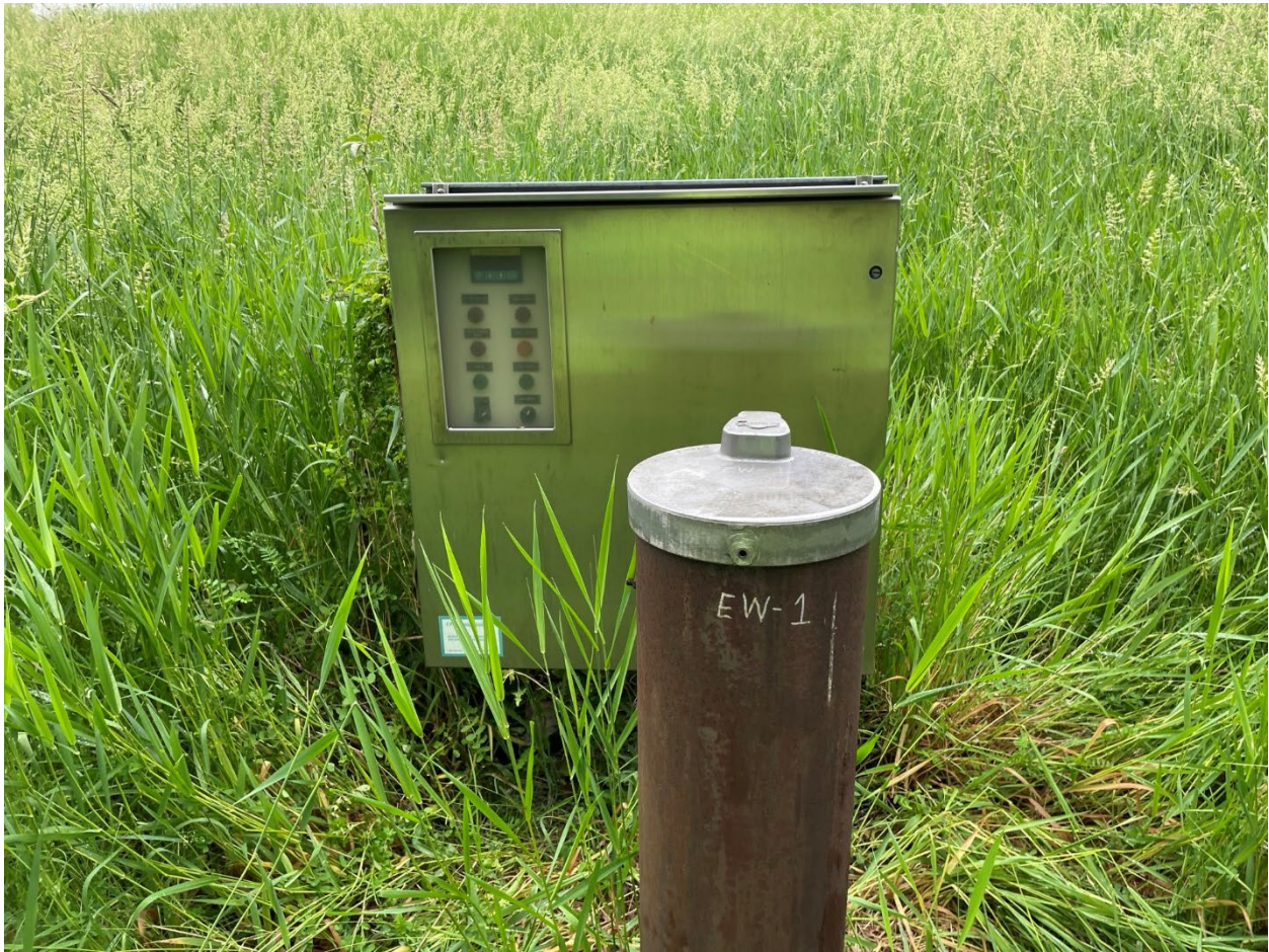
Extraction well (typical, 1 of 3).
