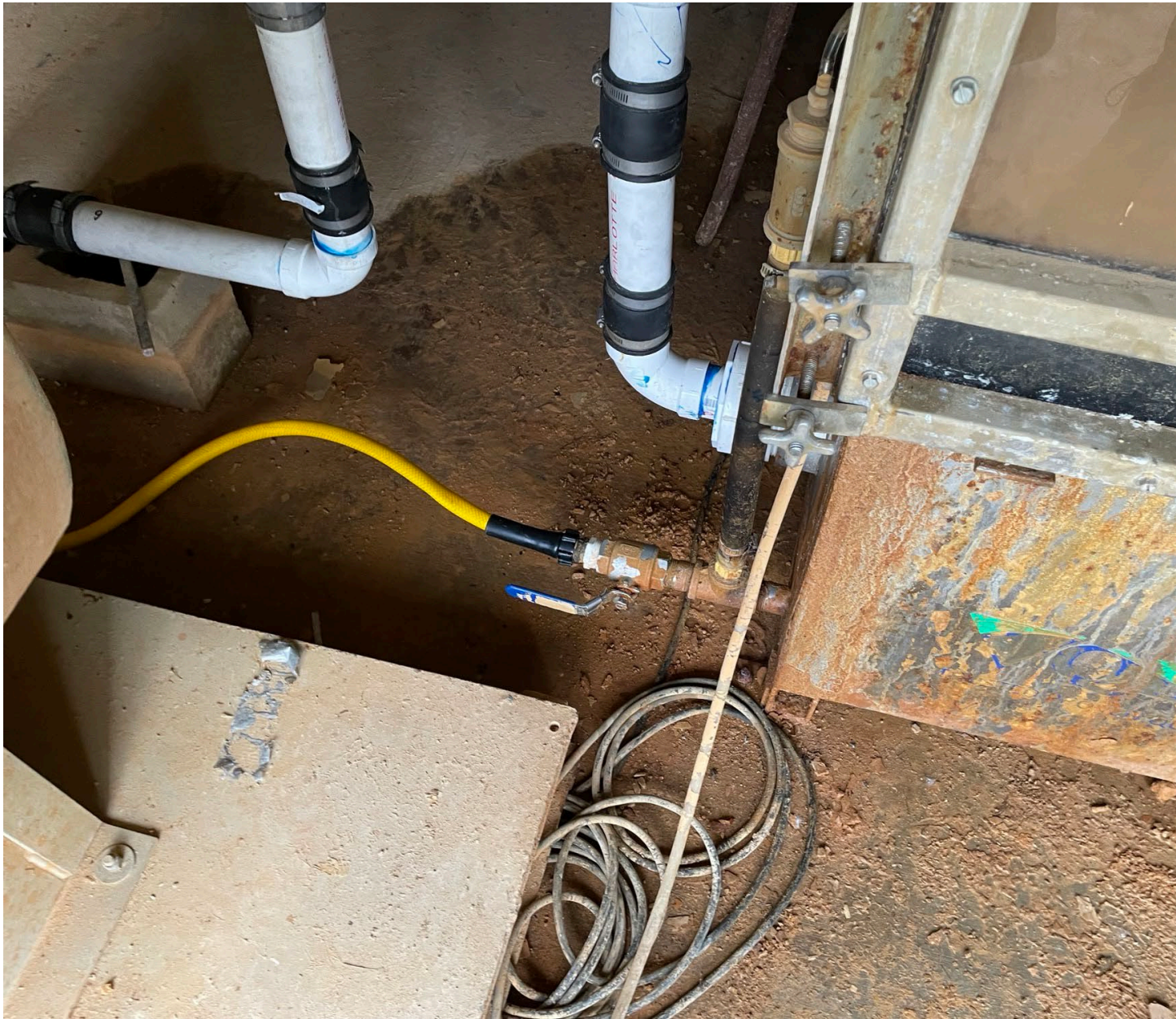
Air stripper cabinet drain hookup (drained prior to removing trays for cleaning).
