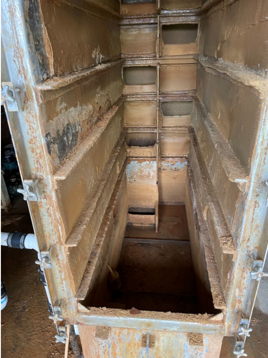
Air stripper cabinet, prior to cleaning.
