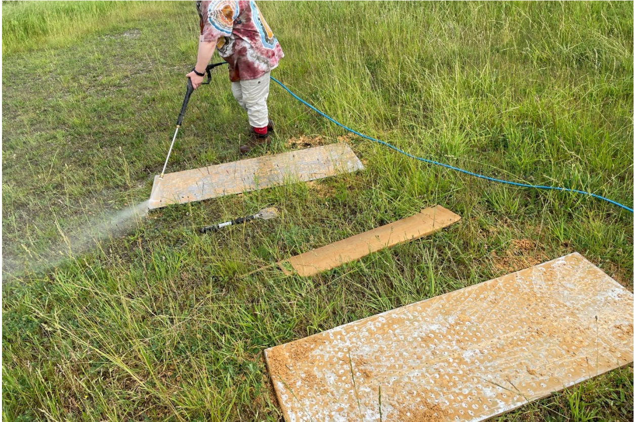
Power washing air stripper trays. Orange/brown accumulation is typical due to high iron groundwater concentrations.
