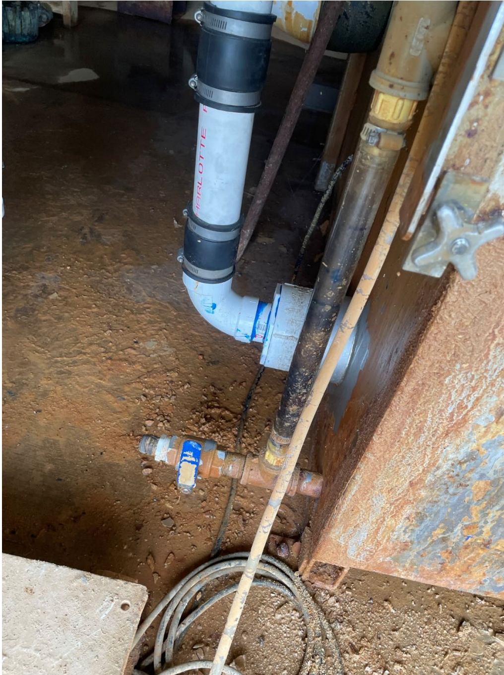
Same as above, outside cabinet connection view.
