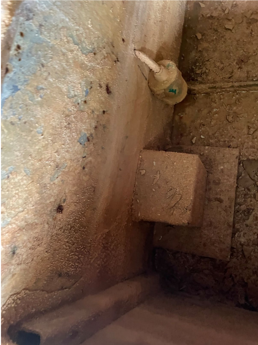
90-degree elbow cover at inside of cabinet. Per AECOM it is difficult to access bottom to clean due to welds.
