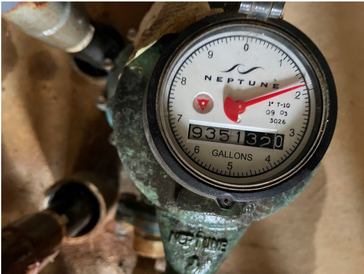
Treatment system flow meter.
