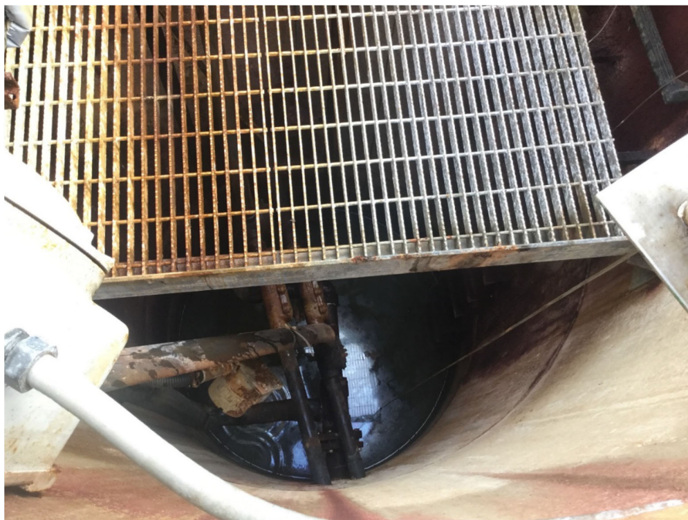
Sheening on the surface of the water at the bottom of Wet Well 6
