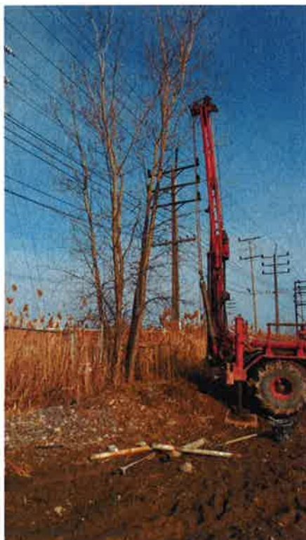
Photo #11: View of the drilling rig near MW-06D and MW-05S and how close it was to the overhead power lines.
