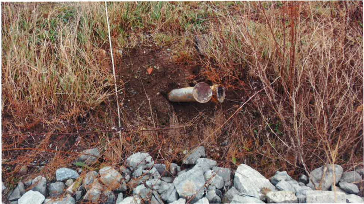
Photo #9: View of the well that was already decommissioned on the Project Site.
