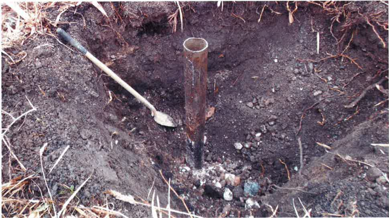
Photo #17: View of MW-06DD – casing has been torched. Waiting on excavator to remove.
