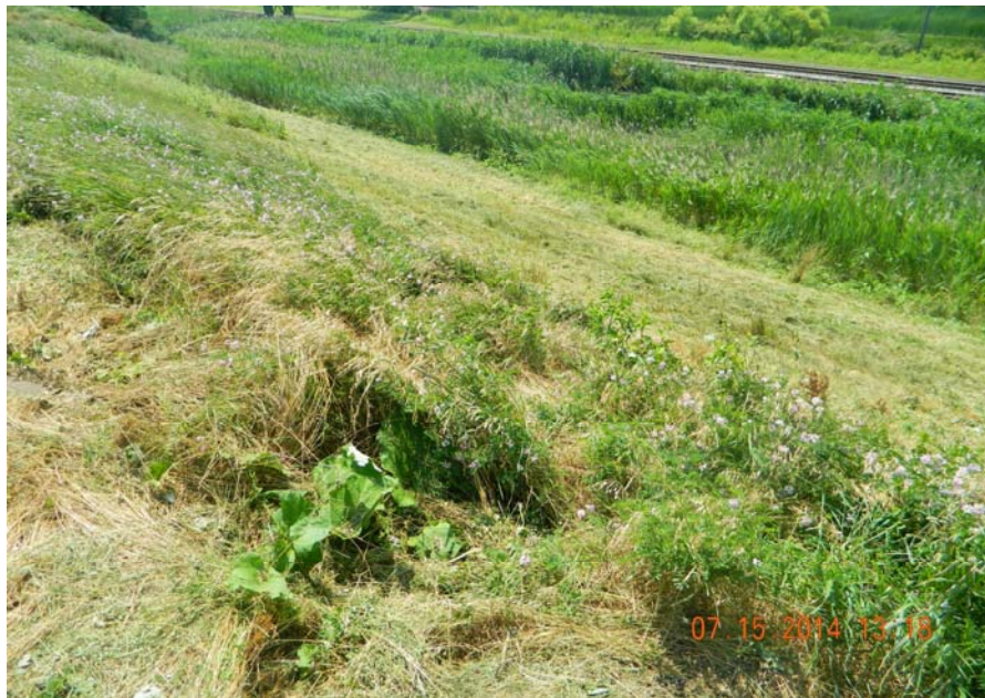
Some erosion along west side of BOF Dust Area where grade becomes steeper
