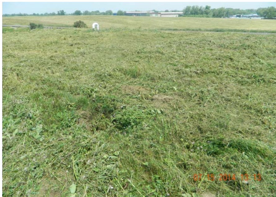
Second smaller hole at top of BOF Dust Area. Approximately 40 feet south of PVC gas vent
