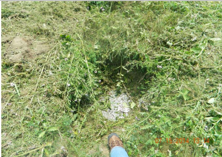
Large hole ~3 feet deep at top of BOF Dust Area with accumulated stormwater. Approximately 40 feet south of PVC gas vent
