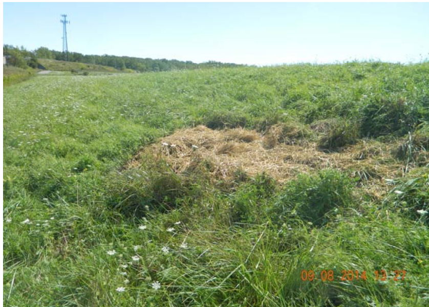
Backfilled, seeded, and mulched animal burrow hole with mud/stone along northeast side of Miscellaneous Debris Area between access road and MW-12B
