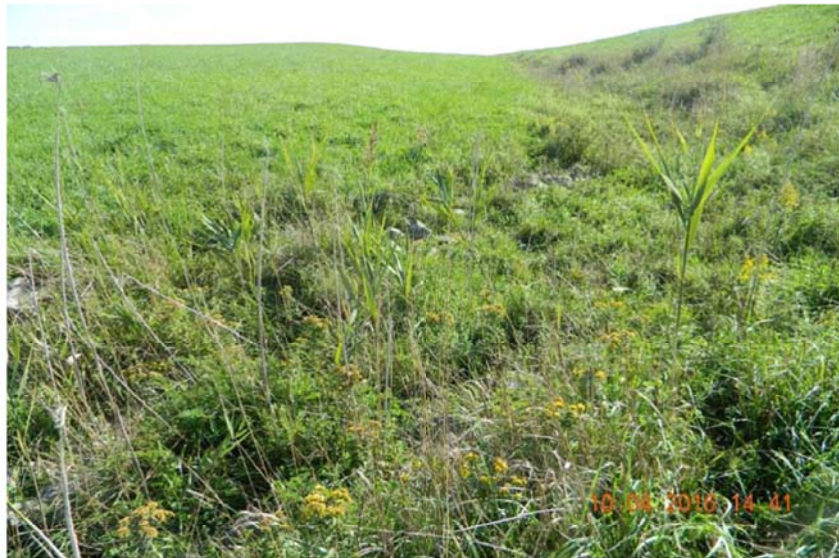
TYPICAL CONDITON OF DOWNCHUTES, TAKEN NORTH OF RAILROAD BRIDGE
