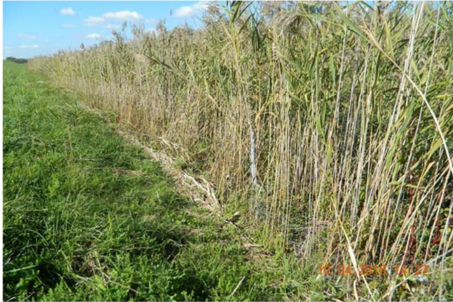
TYPICAL CONDITION AT TOE OF NORTHWEST FACING SLOPE
