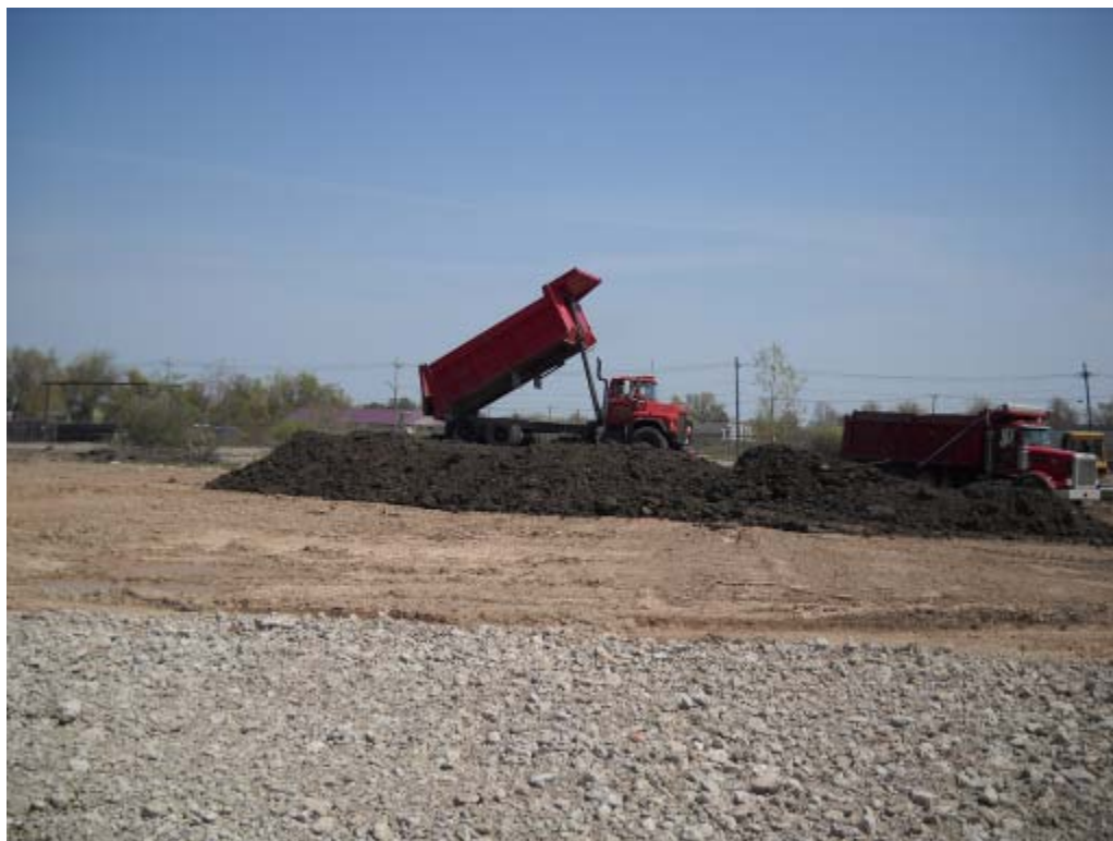
Figure 4 View of Top Soil stockpile at end of day (Looking Southeast) PM
