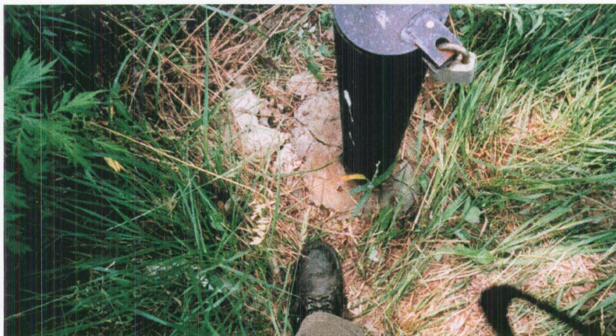
Surface seal on Monitoring Well No GW-2.
