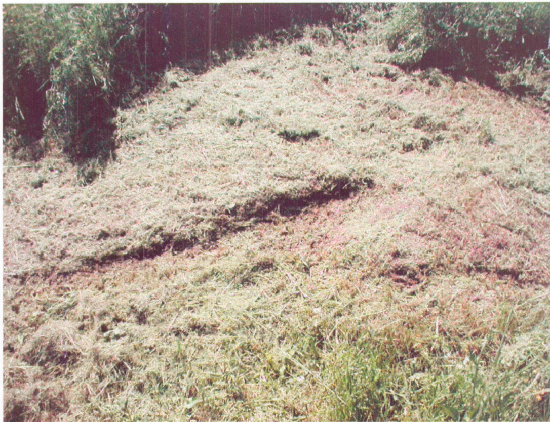
View of area of sloughing
