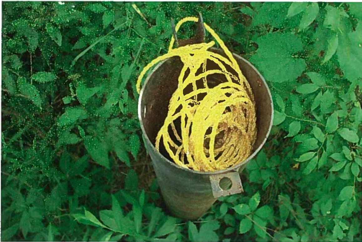
View of GW-2 showing broken top.
