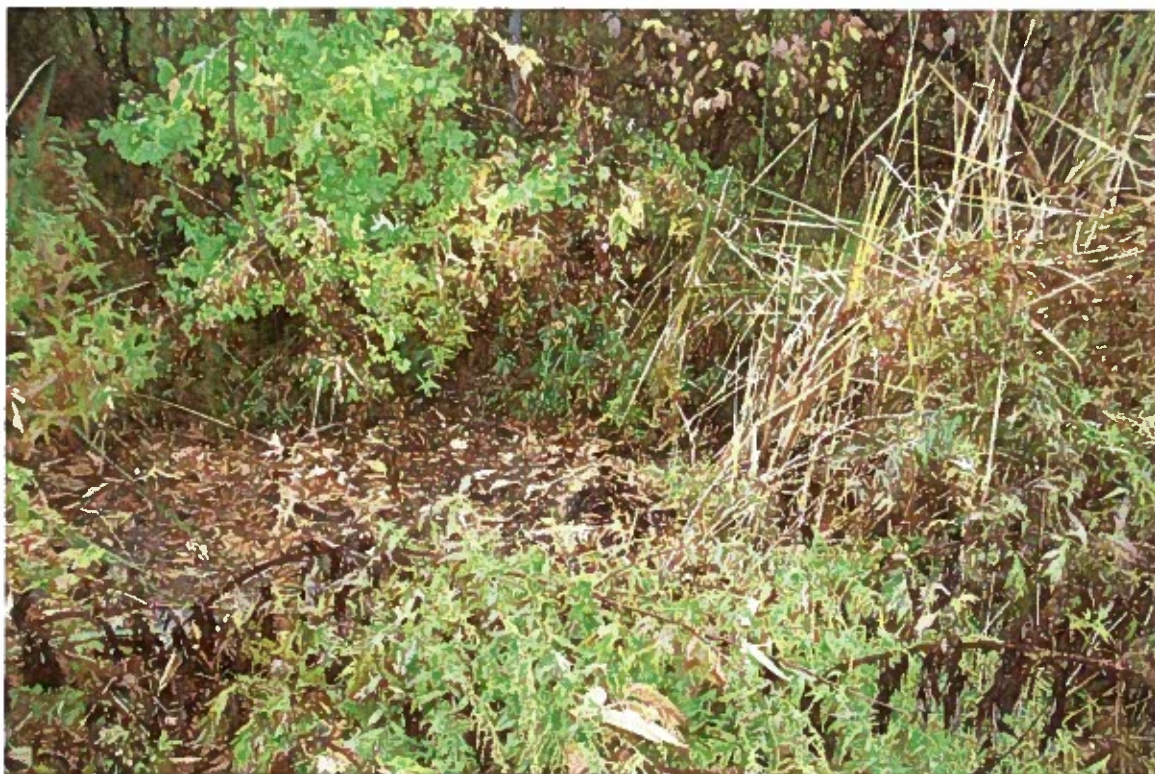
Debris and growth in the drainway.
