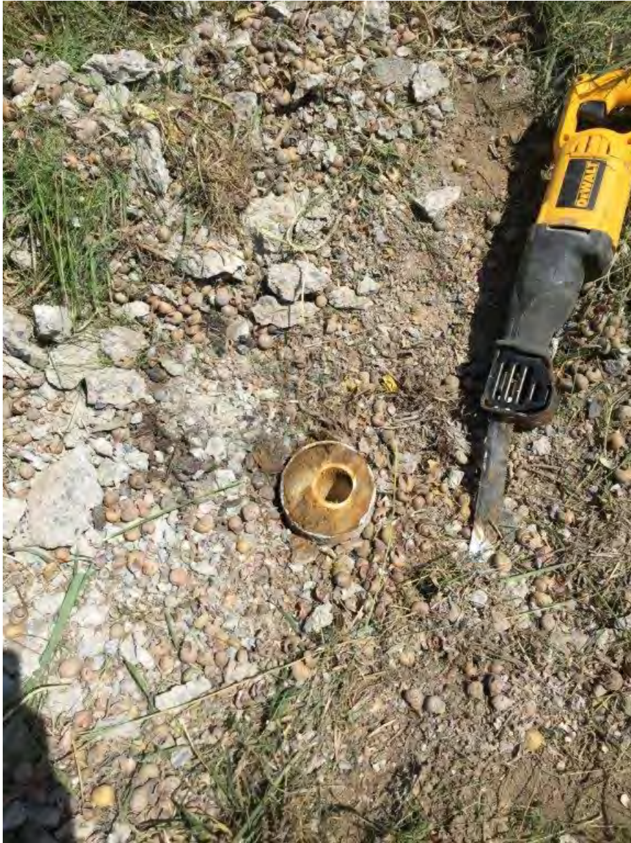
PZ-14 : Piezometer cut below grade
