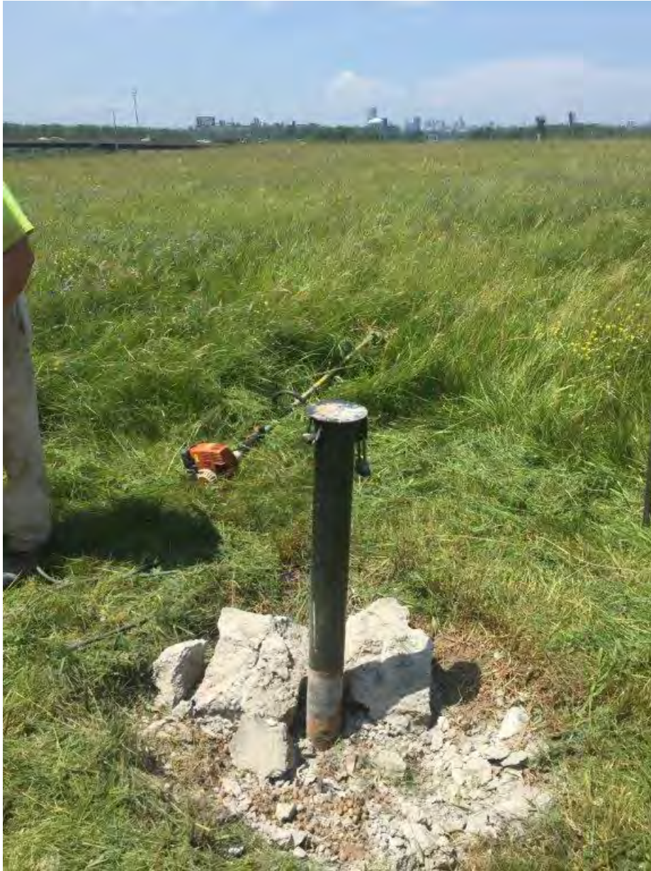
PZ-14 : Concrete pad broken up
