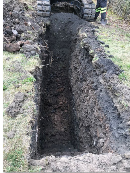
Breeze-rich fill also containing silt, rock, metal, wood, coal, coke, slag, and brick at TP-06-2020.
