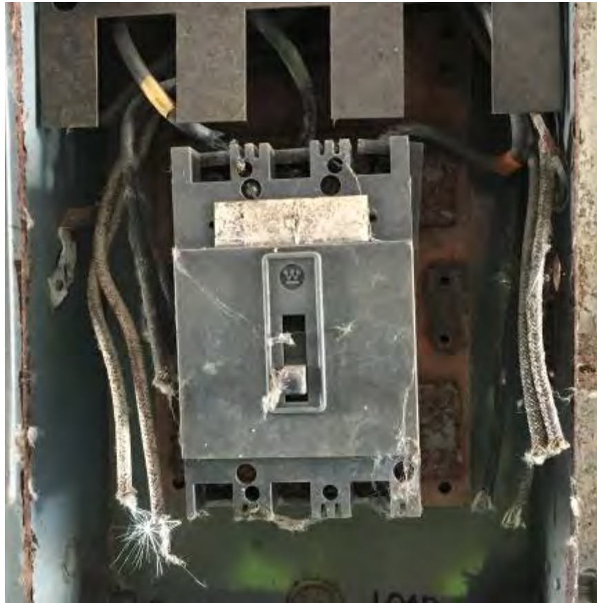
PACM cloth wrap on electrical wiring
