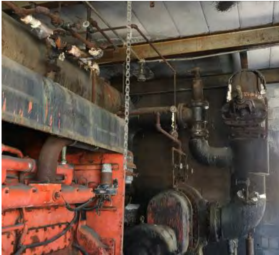
ACM pipe and fitting insulation in poor condition near ceiling and at pump
