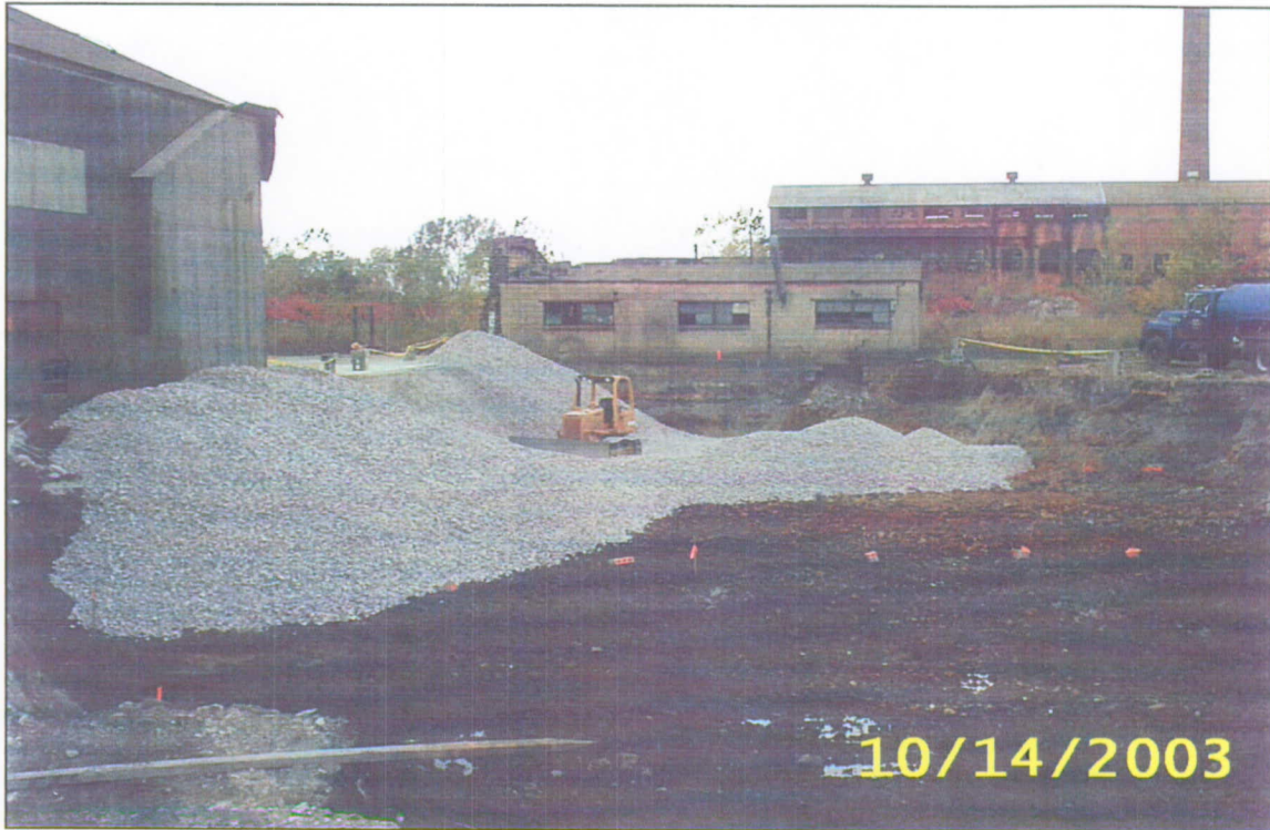
Photograph #5: Placing #3 crushed limestone backfill at the west end of the excavation.
