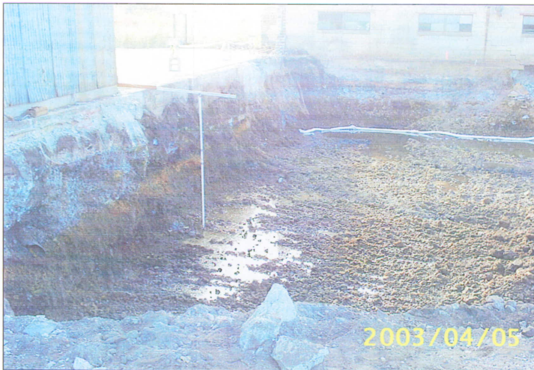
Photograph #2: West end of the excavation, with some water at the floor. (Note: the camera date stamp should read 10/9/2003)
