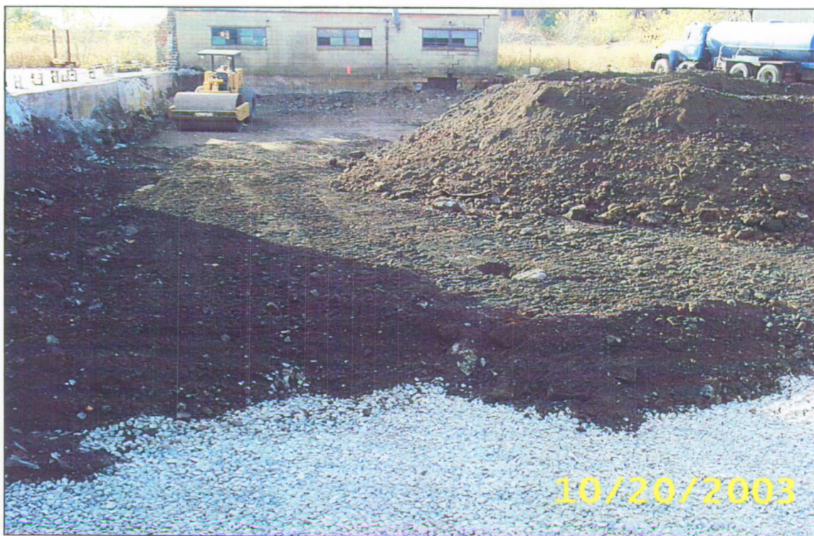
Photograph #13: Reusable soil being compacted at the west end of the excavation.
