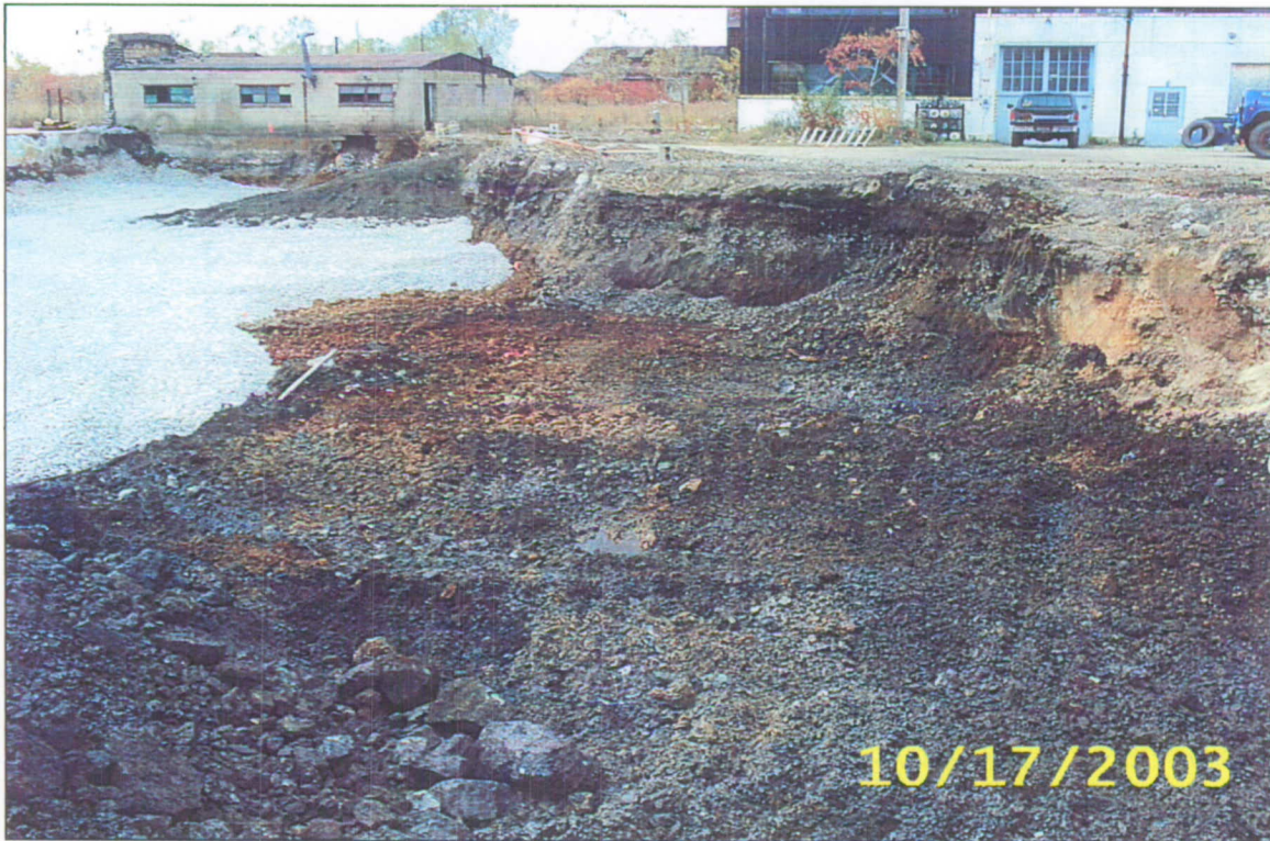
Photograph #12: North wall of the excavation, with reusable soil ramp at west end.
