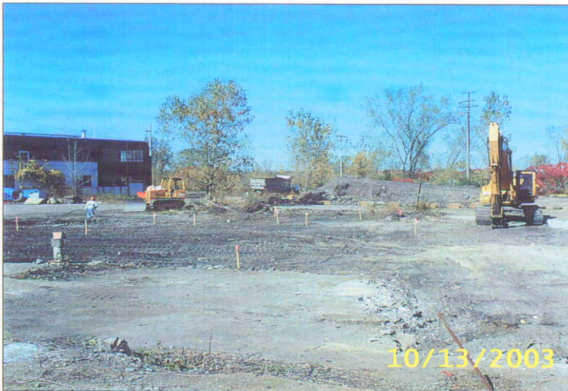
Photograph #4: Proposed eastern limits of excavation with concrete removed. (Note: the camera date stamp should read 10/13/2003)
