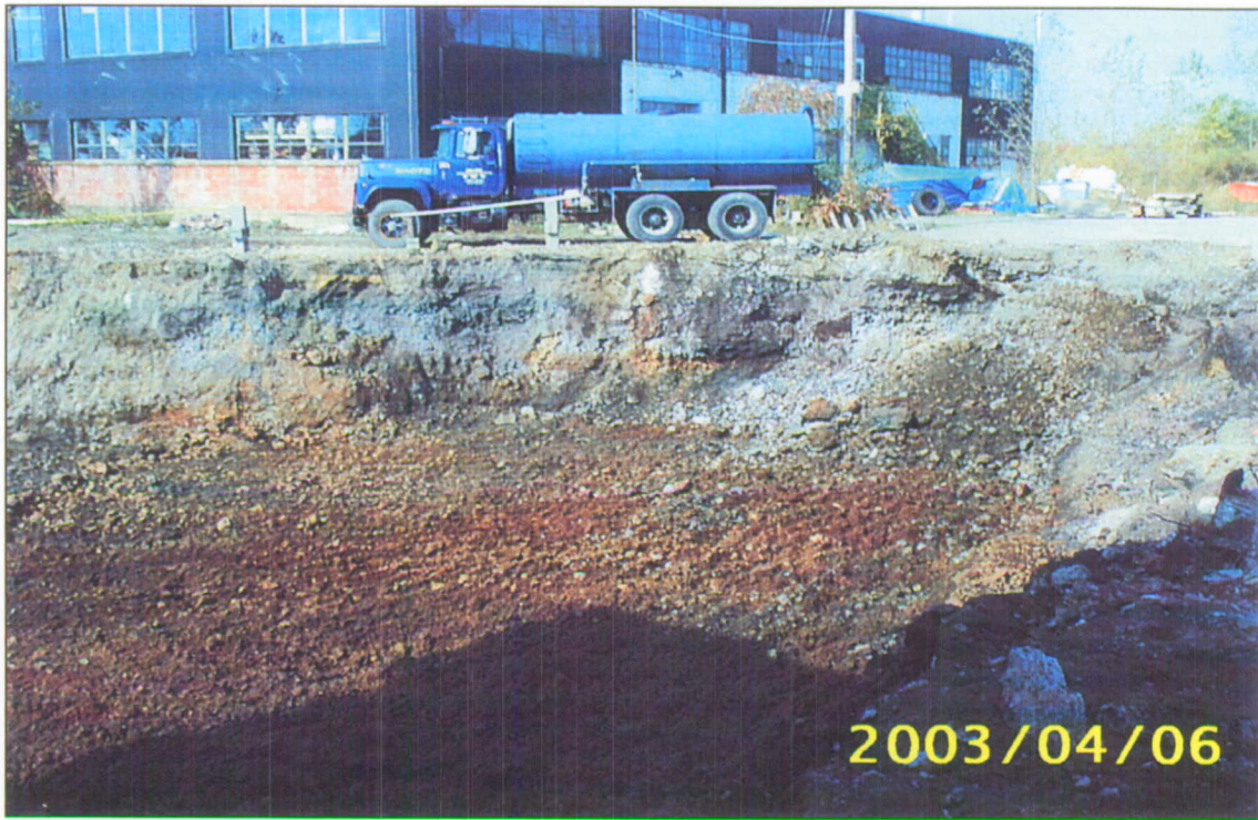
Photograph #3: North wall of the excavation. (Note: the camera date stamp should read 10/10/2003)
