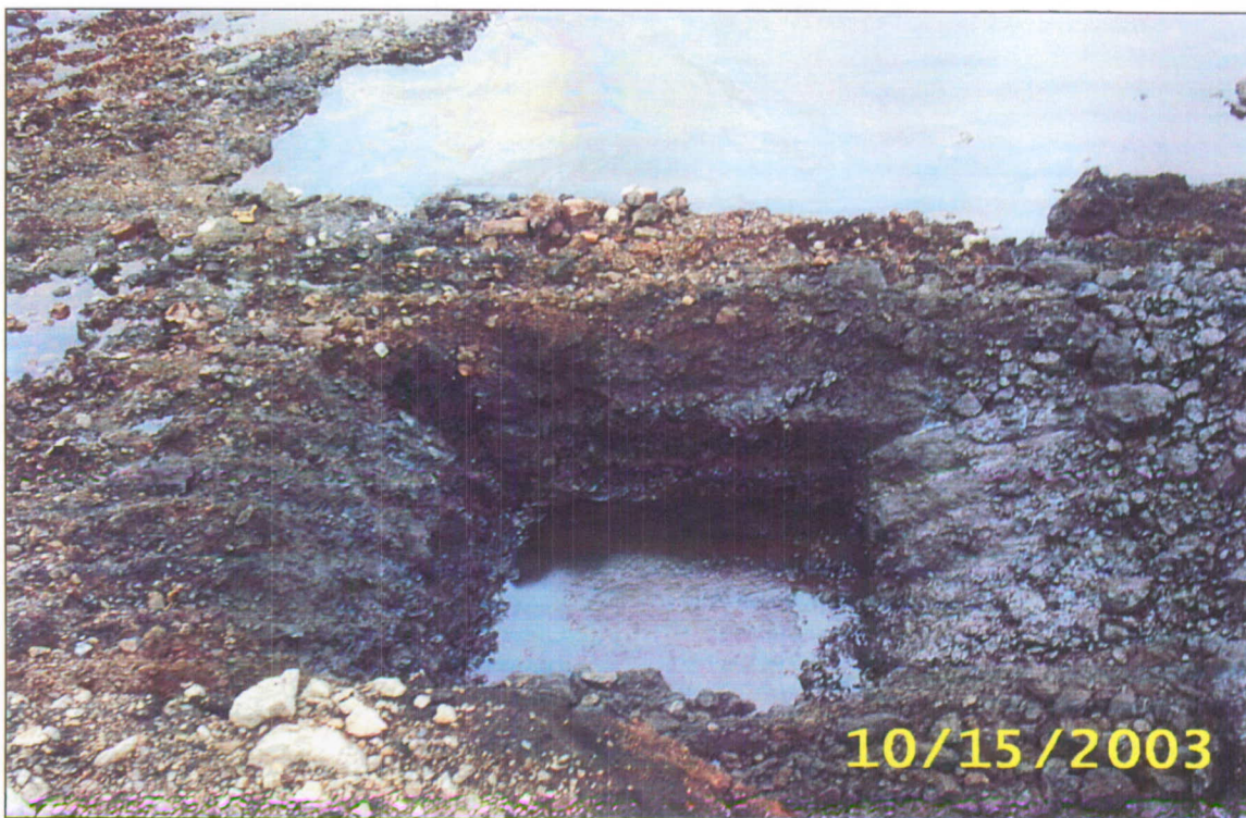
Photograph #9: Test pit adjacent to hazardous waste area to delineate extent of waste. This material was removed.
