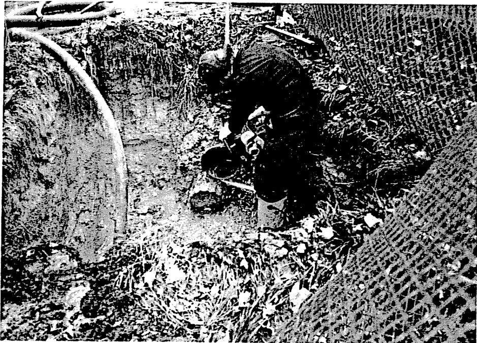
Photo #2 Cutting concrete plug out of 8 inch drain to enable area drainage. Photo looks north.
