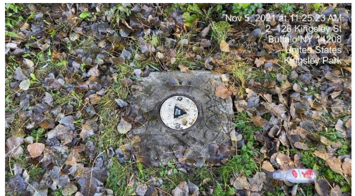
Monitoring Well MW-6
