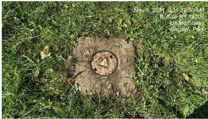
Monitoring Well MW-1
