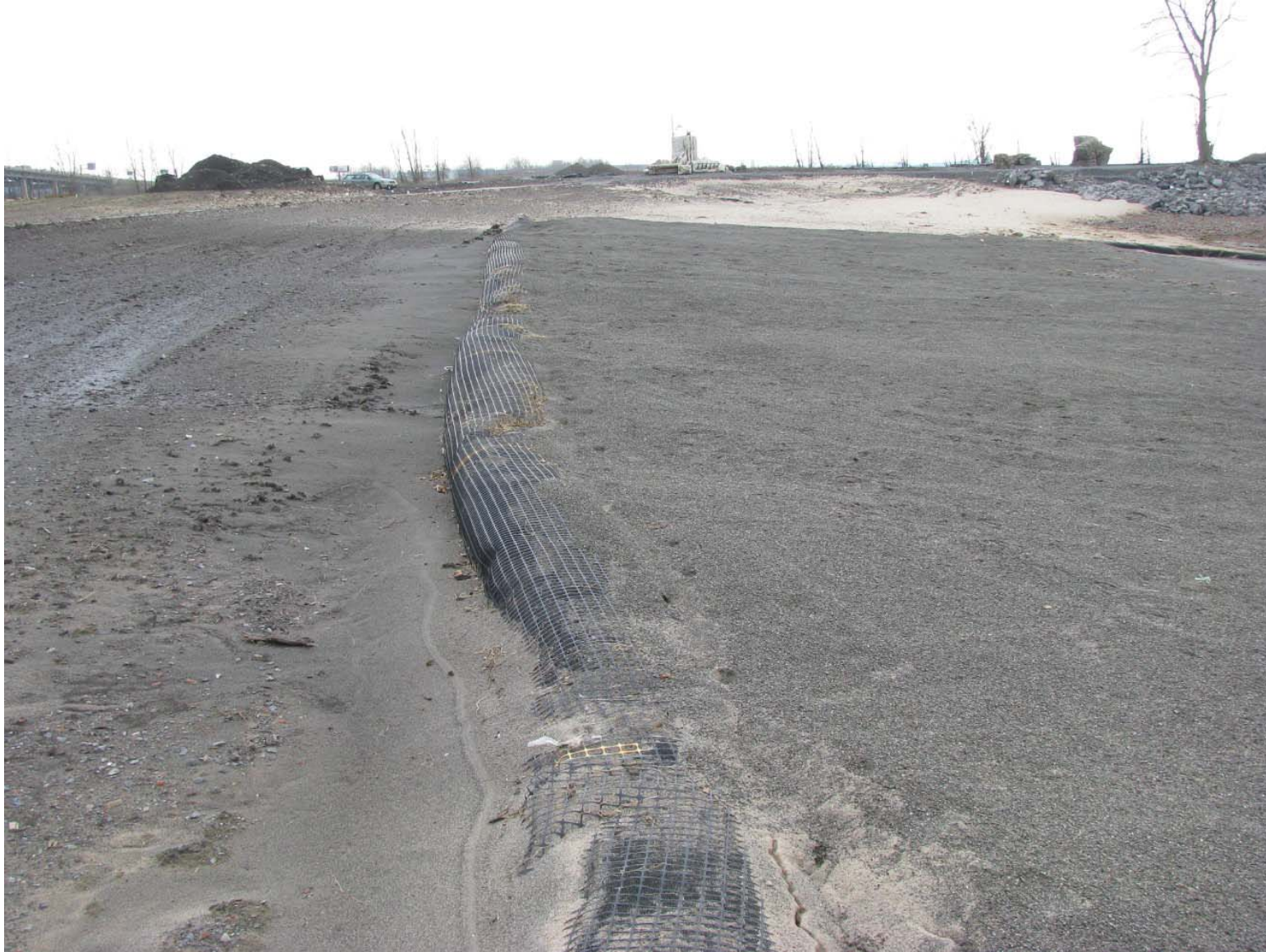
NYPA Parcel Photo 6: Looking south along the inland edge restraint – note the evidence of minor wave overtopping.
