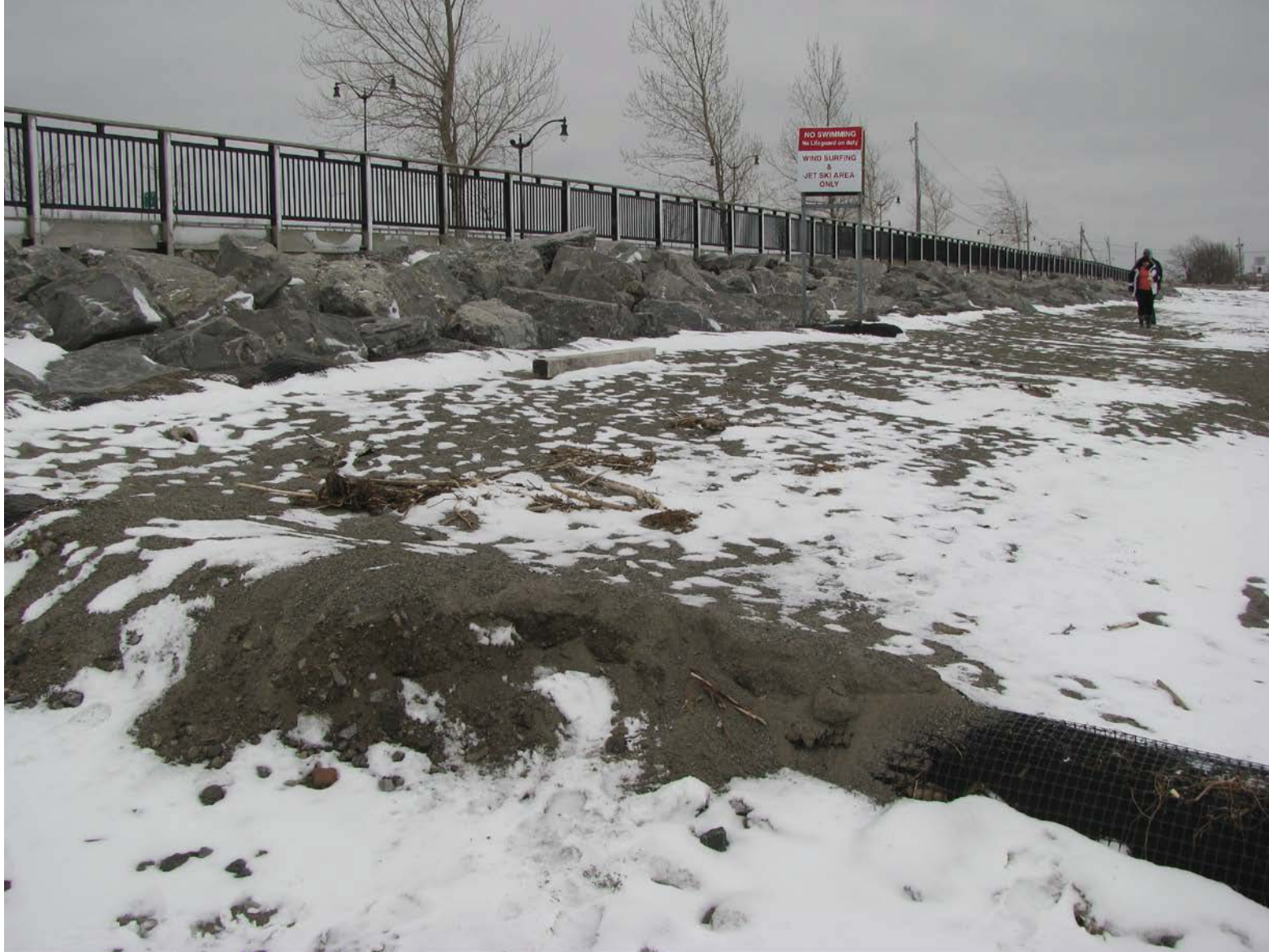
Gallagher Beach Photo 5 Looking southeast at the top of the test area. Note the sand mound that someone has placed over the edge restraint in the foreground. There is no apparent damage to the edge restraint.
