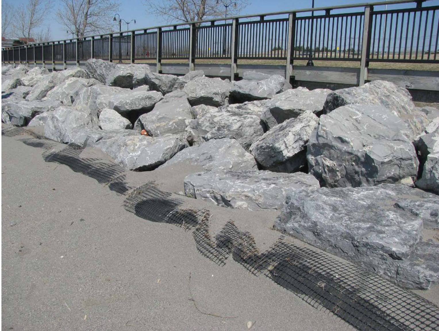
Gallagher Beach Photo 10: Looking north at the wind-blown sand in the upslope riprap
