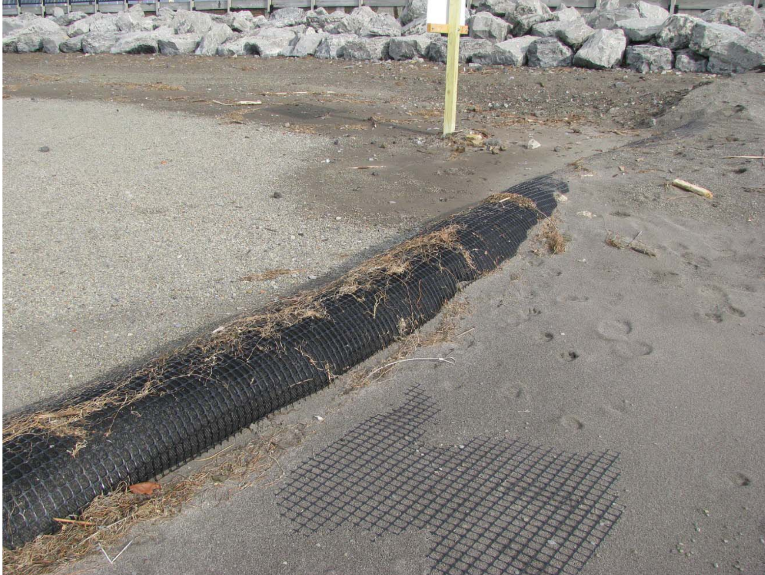
Gallagher Beach Photo 11: Northeast corner of test area showing exposed lock-down netting, loose anchor, and elevation difference between lock-down netting on the inside of the test area and “existing grade” on the outside.
