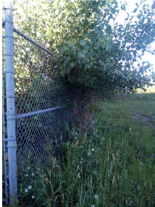
Photo No. 7 – Vegetation growth within drainage swale along fence line.
