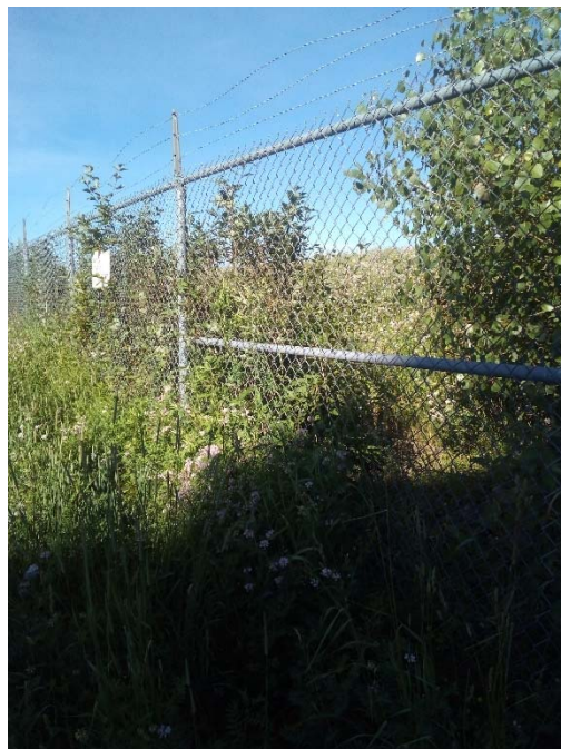
Photo No. 8 – Vegetation growth within drainage swale along fence line.
