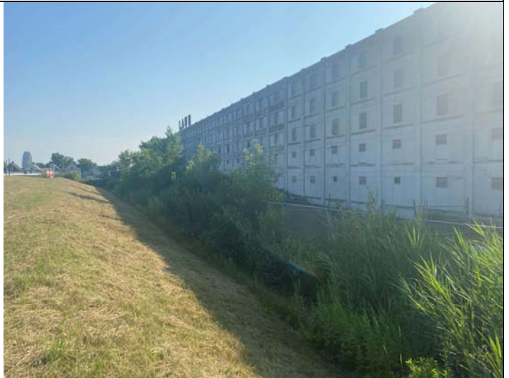
Vegetative growth along the eastern perimeter
