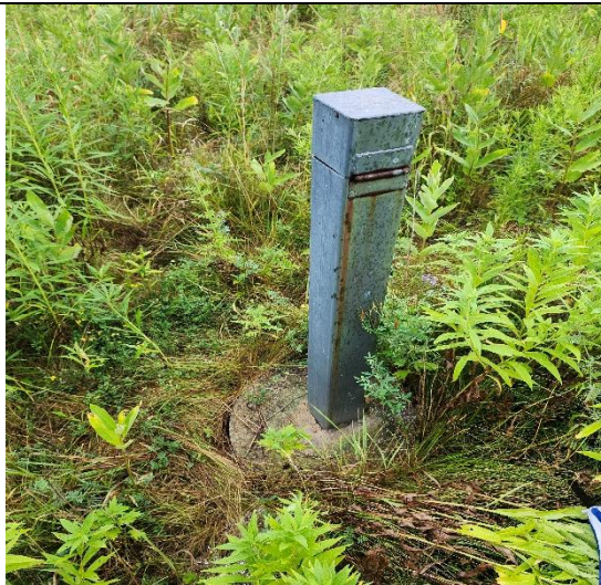
Typical Monitoring Well
