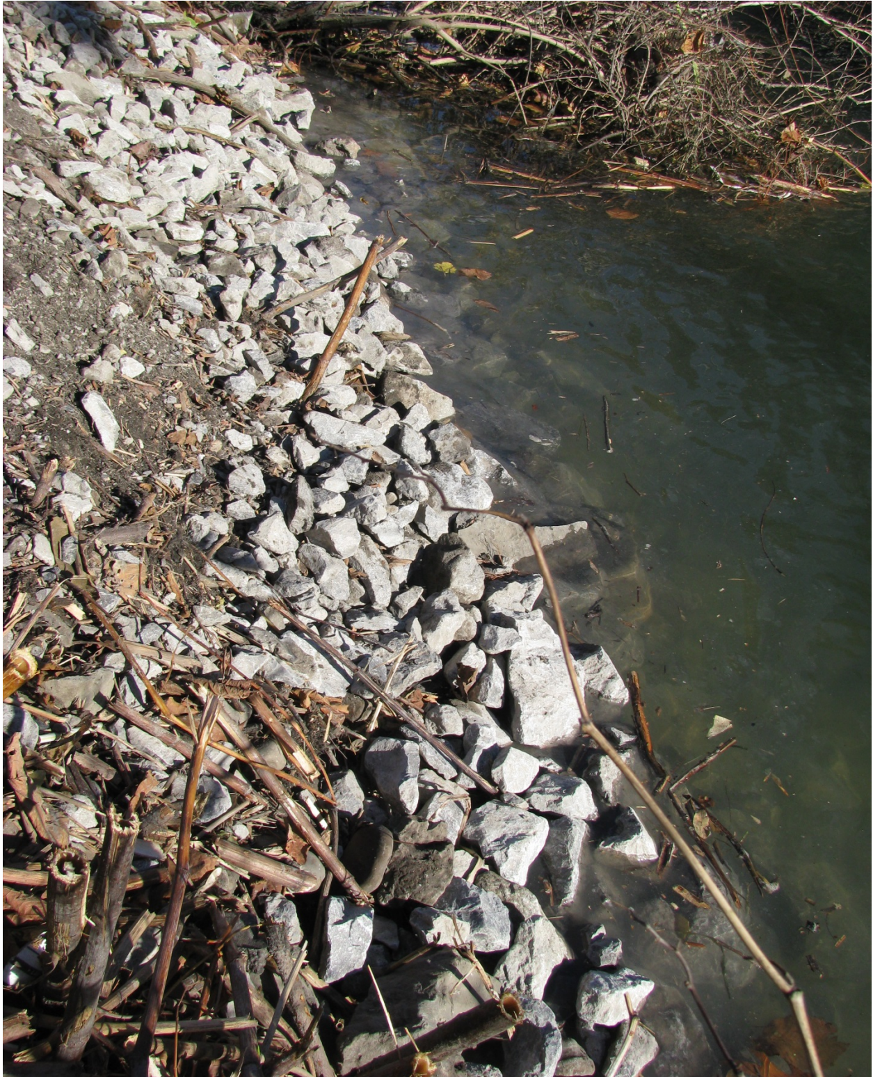
Maintenance stone placed near water's edge at Area 1.
