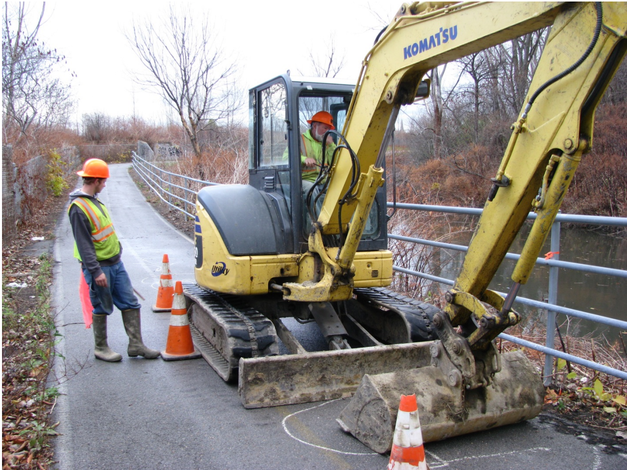
Rubber-tracked equipment used by the Contractor to clear vegetation and place and/or position stone.
