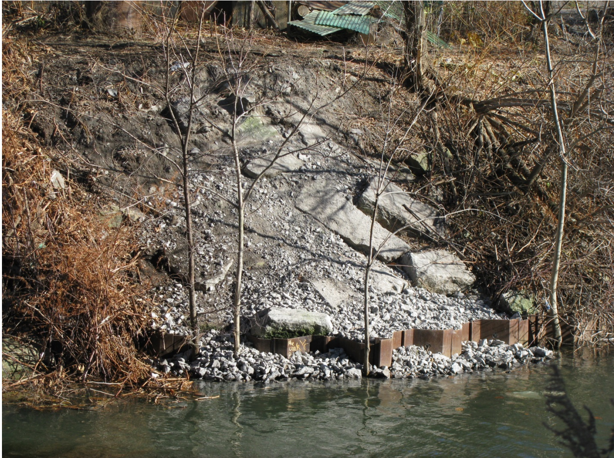
Completed maintenance activity at Area 4 (located in front of sheet pile wall). Apparent bare soils will be monitored for erosion in future site inspections.
