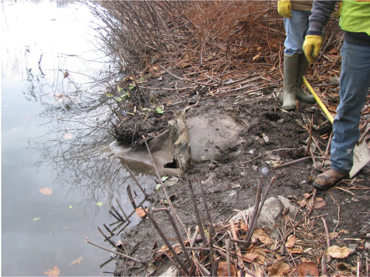
Damaged textile at Area 5. The textile had torn, and was further slit to eliminate bridging over missing stone/soil below, and to allow it to lie flat beneath replaced armor.
