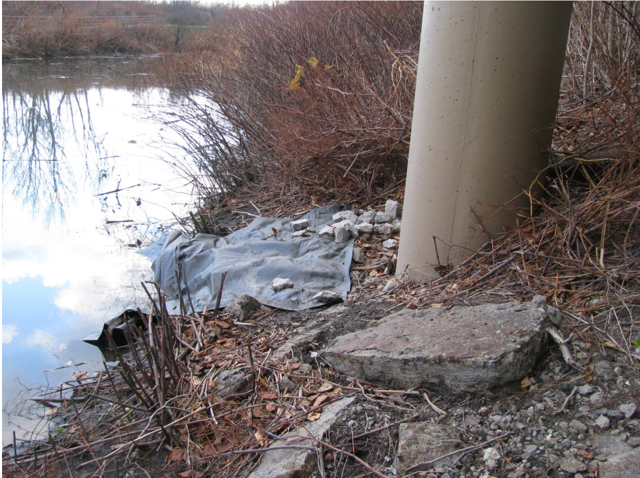
Geotextile patch placed to cover the torn/slit existing textile at Area 5. The replacement textile was affixed to the underlying soil with pins.
