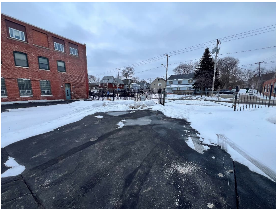
Photograph No. 4: Parking lot surface conditions. View is east.
