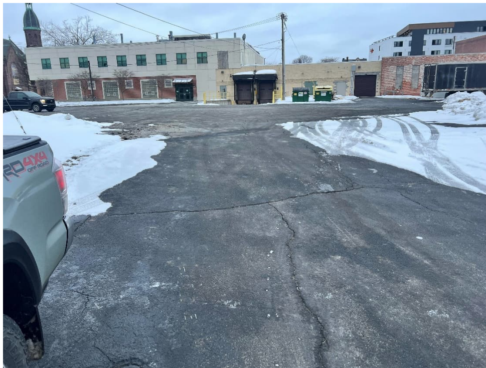
Photograph No. 3: Parking lot surface conditions. View is west.
