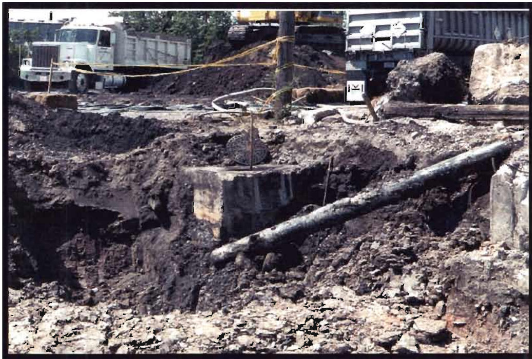
Photo 14: View of Sump Near Southeast Corner of Building [View to Northwest]
