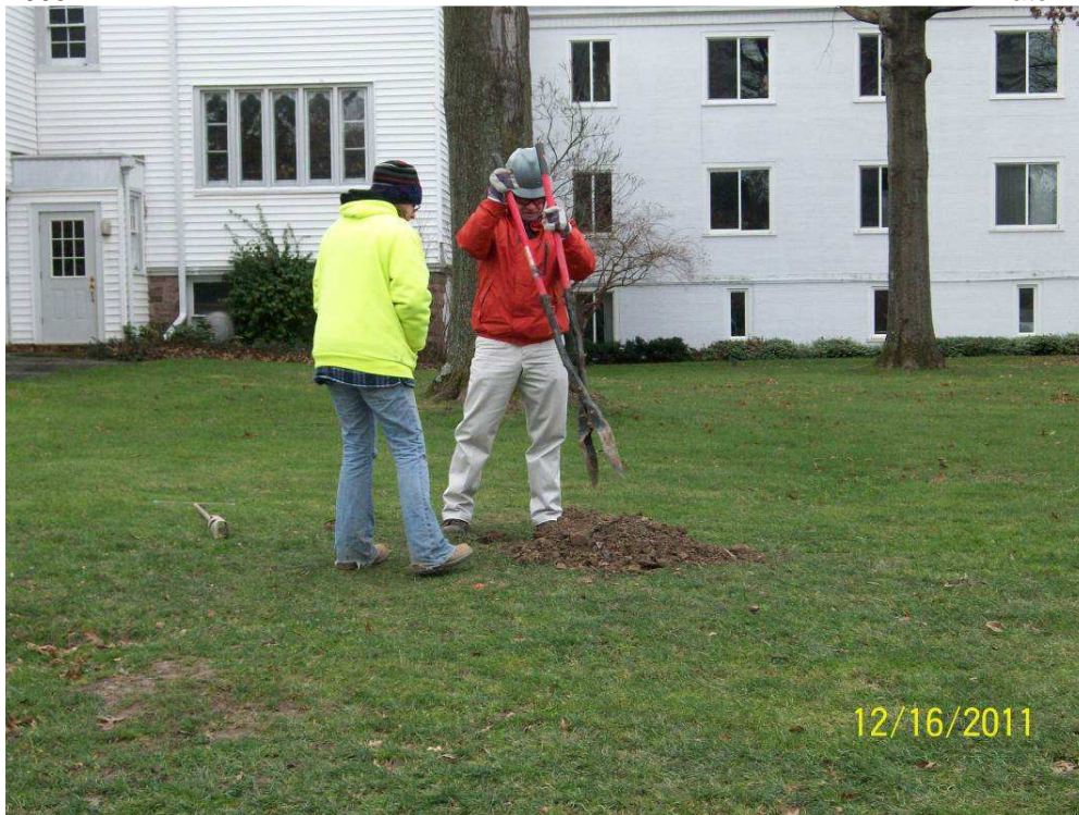
Figure 1: View of Hand Excavation to 5' for Utility Clearance at EE-3 (Looking South AM)
