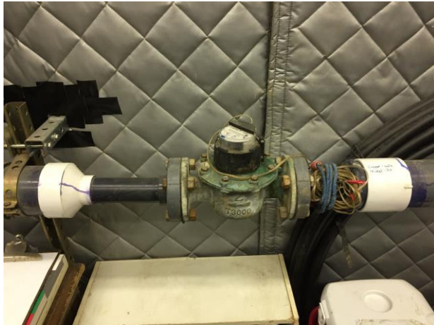
The Effluent Meter showing the pipes being downsized from the 4" SCH-40 PVC.
