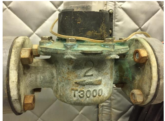
Close side view of the Effluent Meter.
