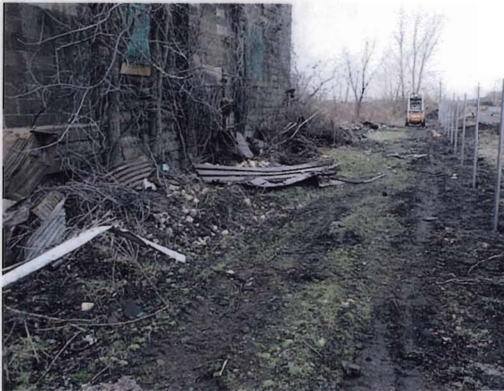
Lackawanna Foundry Site - Condition of Buildings along eastern edge of Site, during fence installation.
