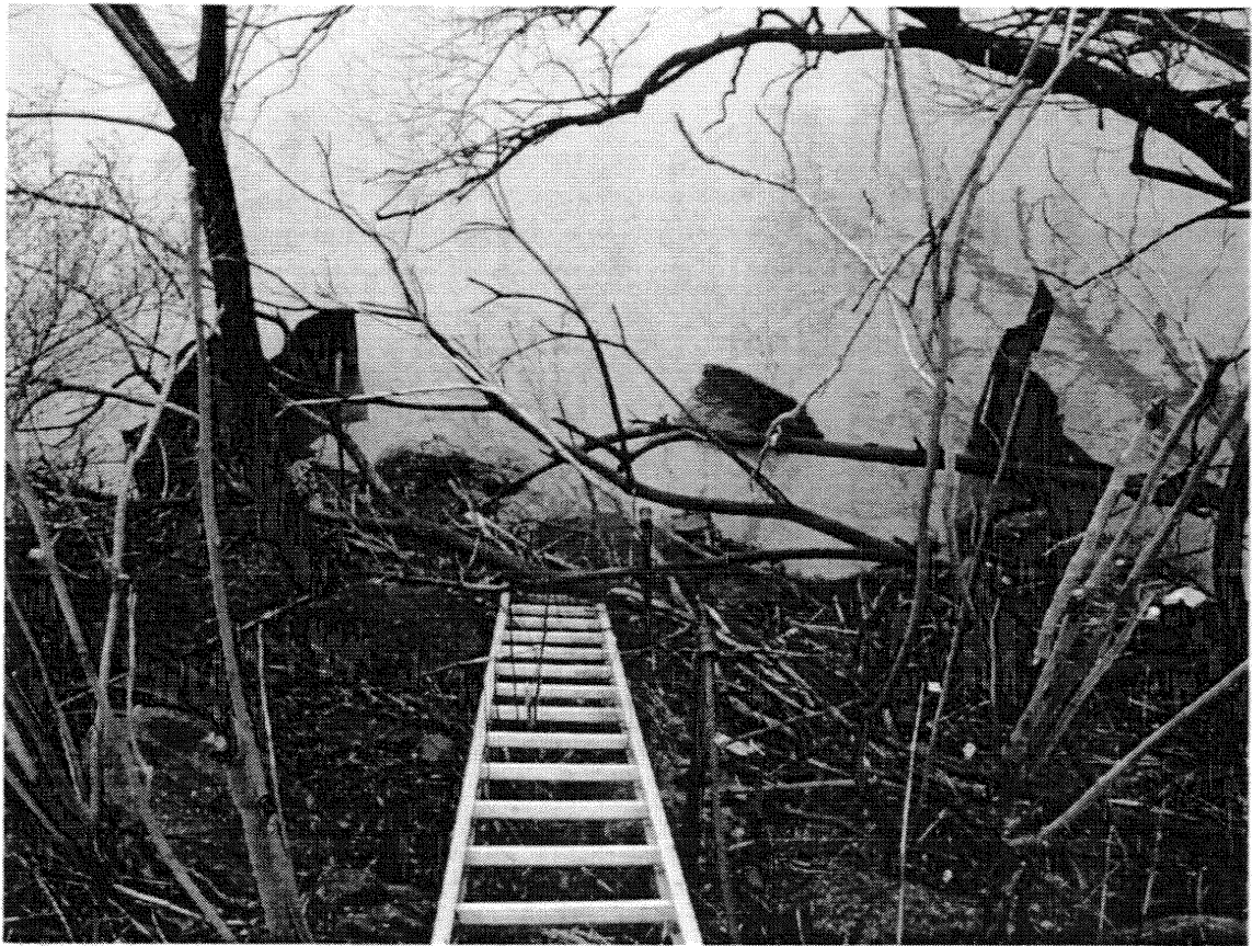
) Photo 2 – River Bank showing poor condition. Date: 04/14/04
