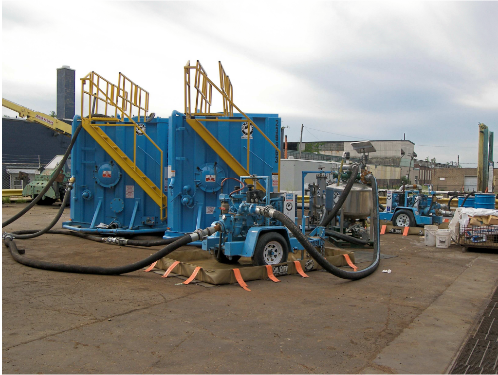
Picture 9 – View of the water treatment system.
