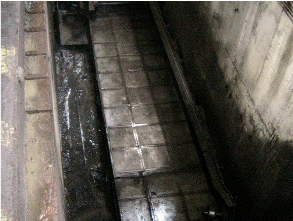
Picture 4 – Looking north across stainless steel screen and tank bottom.
