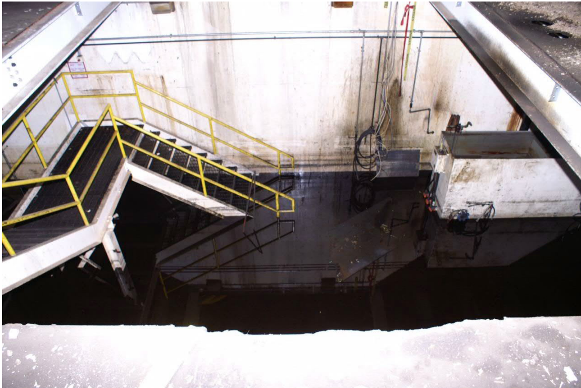
Photograph 3 Pit Containing Oily Substance and Wastewater Circa 2009 (Before GM Bankruptcy)
