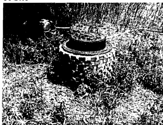
Manhole near 5,000,000-gallon AST
