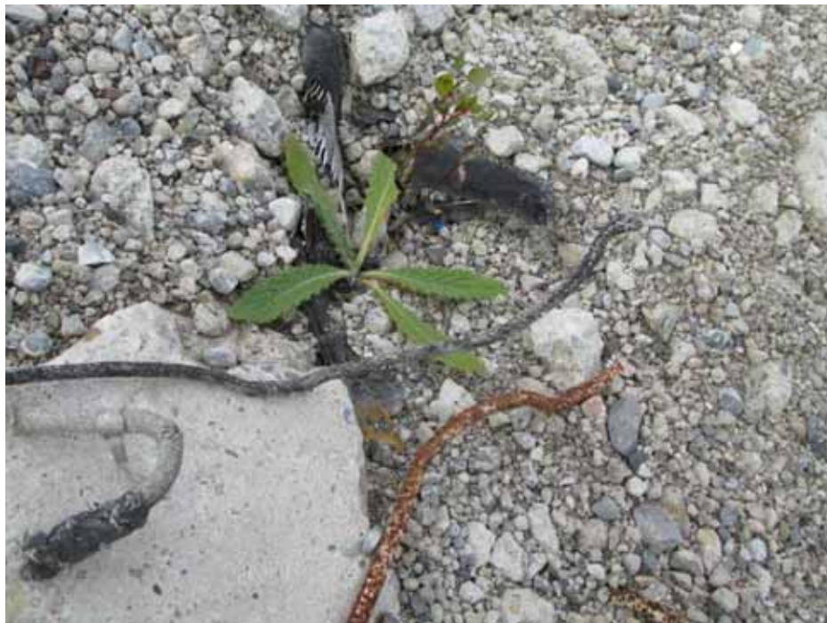
Photo 4: 11/5/13 – Insulated wire (typical).
