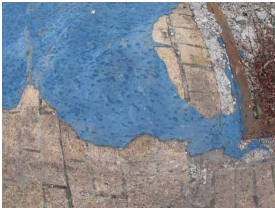
Photo 37: 11/11/13 – Blue thick floor coating (non-ACM).
