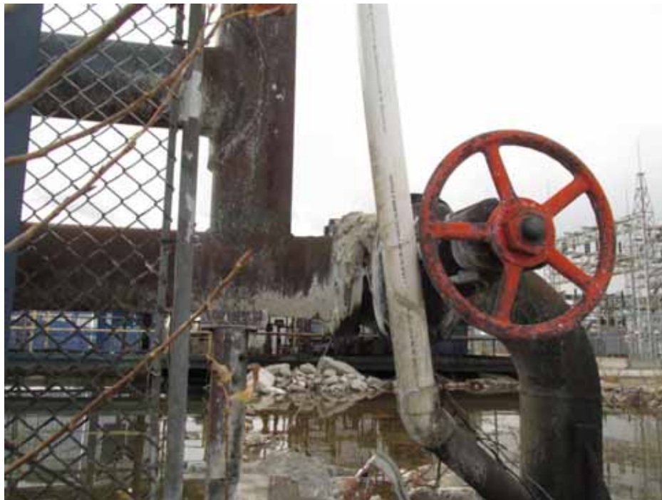
Photo 12: 11/8/13 – White mud insulation (ACM) in grid R4.
