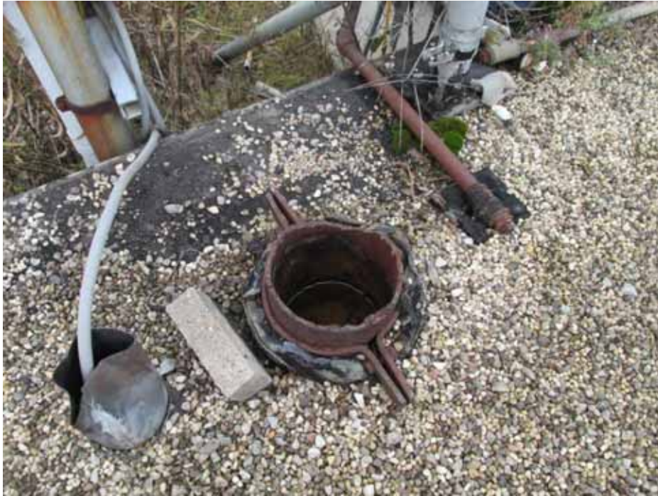
Photo 15: 11/8/13 – Grey penetration flashing (ACM) in grid S4.
