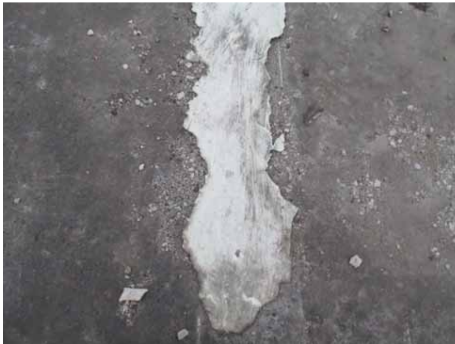
Photo 9: 11/6/13 – Grey/Lt grey floor leveling compound/coating (ACM).
