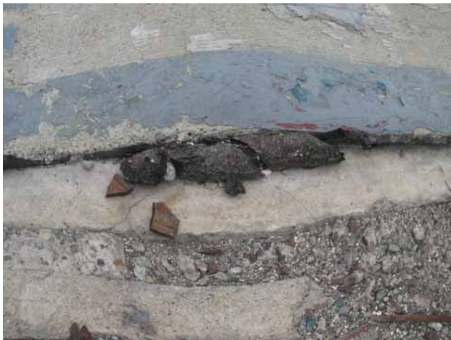
Photo 33: 11/11/13 – Black expansion joint (ACM-typical).
