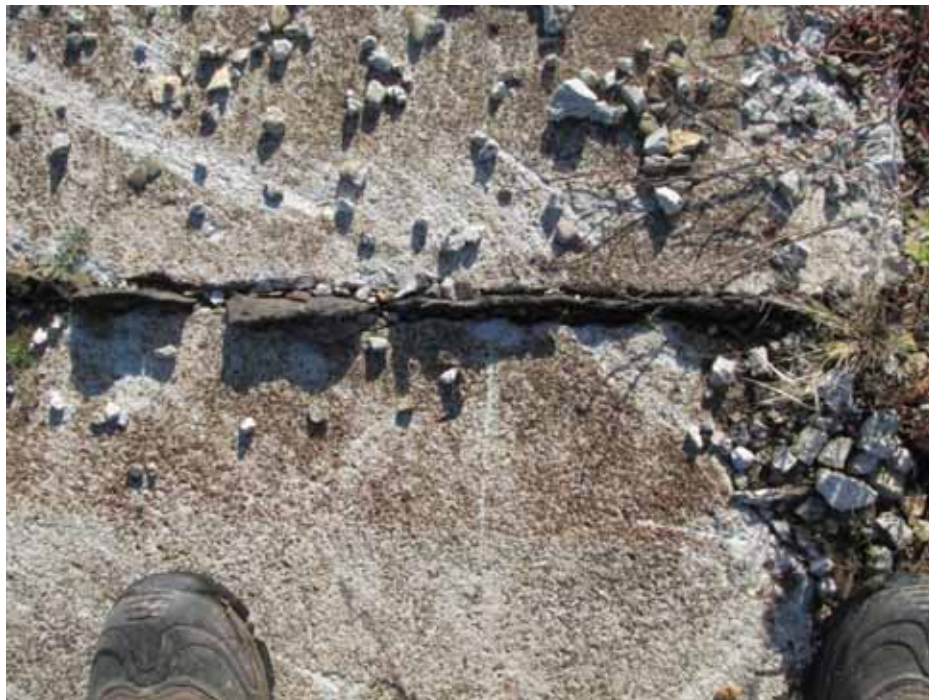
Photo 10: 11/6/13 – Black expansion joint (ACM-typical).
