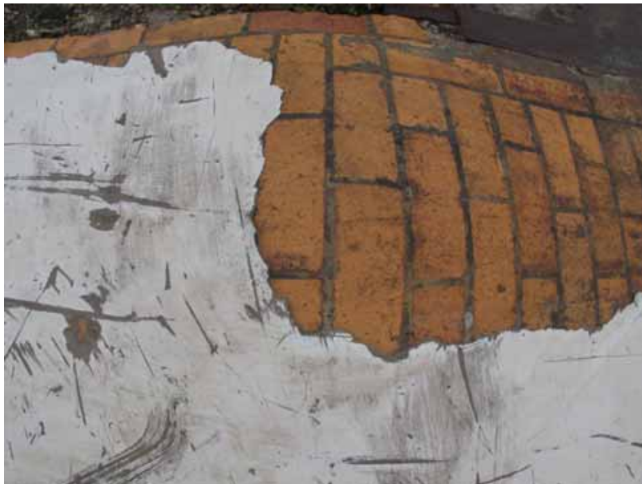
Photo 42: 11/11/13 – Grey/Lt grey floor leveling compound/coating (ACM).
