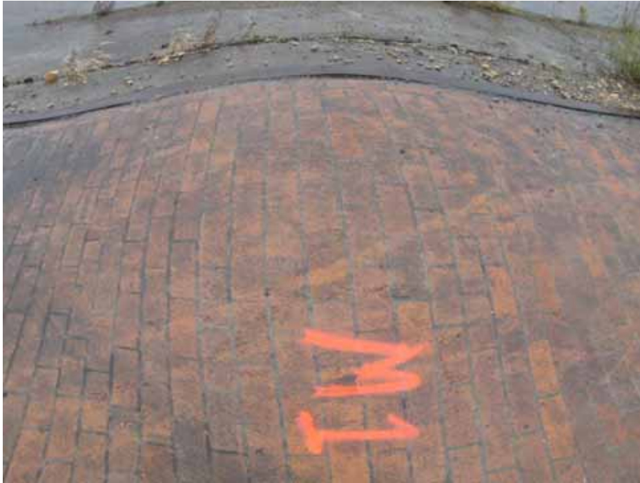
Photo 47: 11/11/13 – Red bricks in grid M1.
