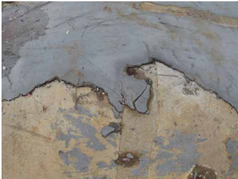
Photo 28: 11/11/13 – Blue thick floor coating (non-ACM).
