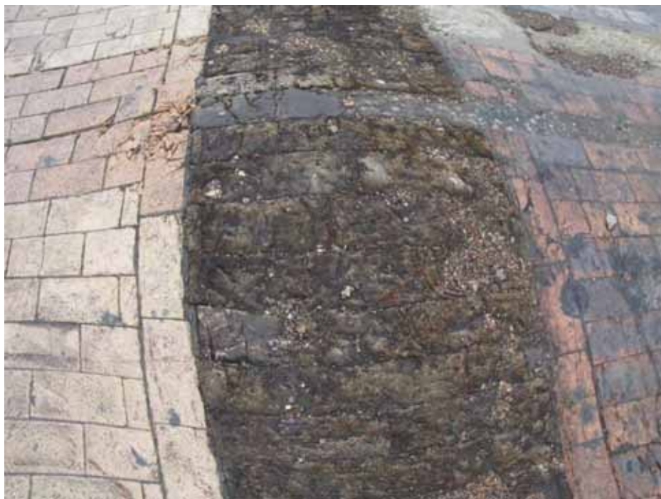
Photo 40: 11/11/13 – Coated wood joints in floor (not surveyed).
