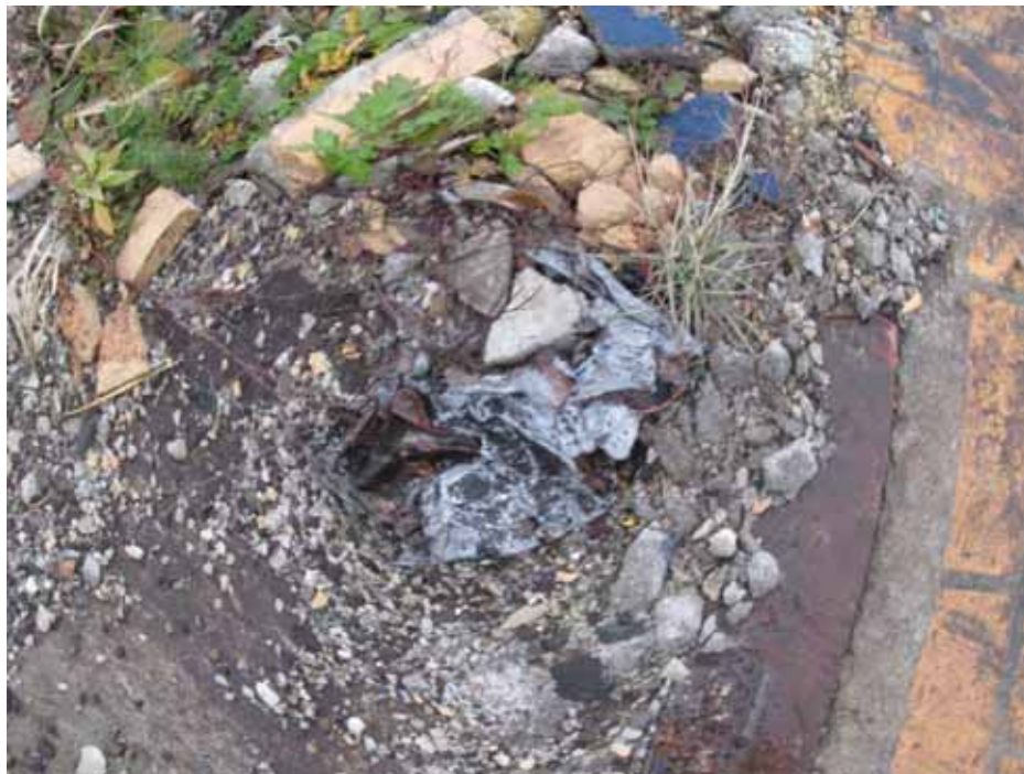
Photo 41: 11/11/13 – Galbestos (ACM) in debris pile.
