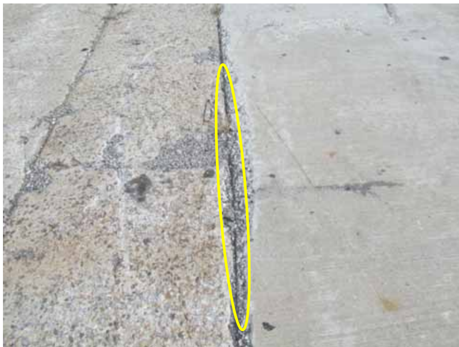
Photo 3: 11/5/13 – Black expansion joint (ACM-typical).
