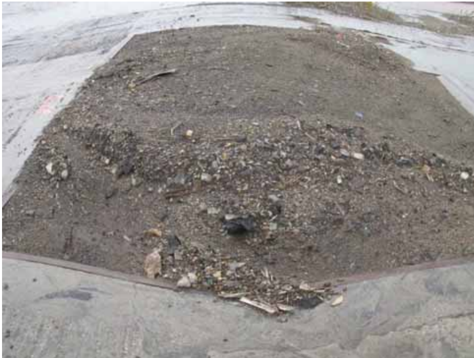
Photo 48: 11/11/13 – Pits filled with debris containing ACM roofing material throughout (typical).
