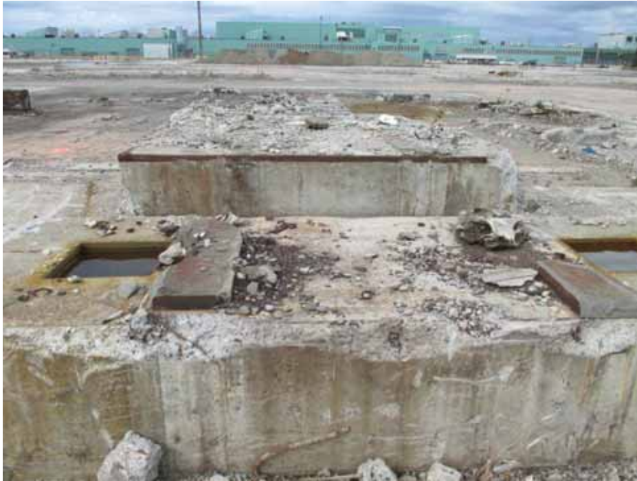
Photo 7: 11/6/13 – Concrete footers with miscellaneous debris.
