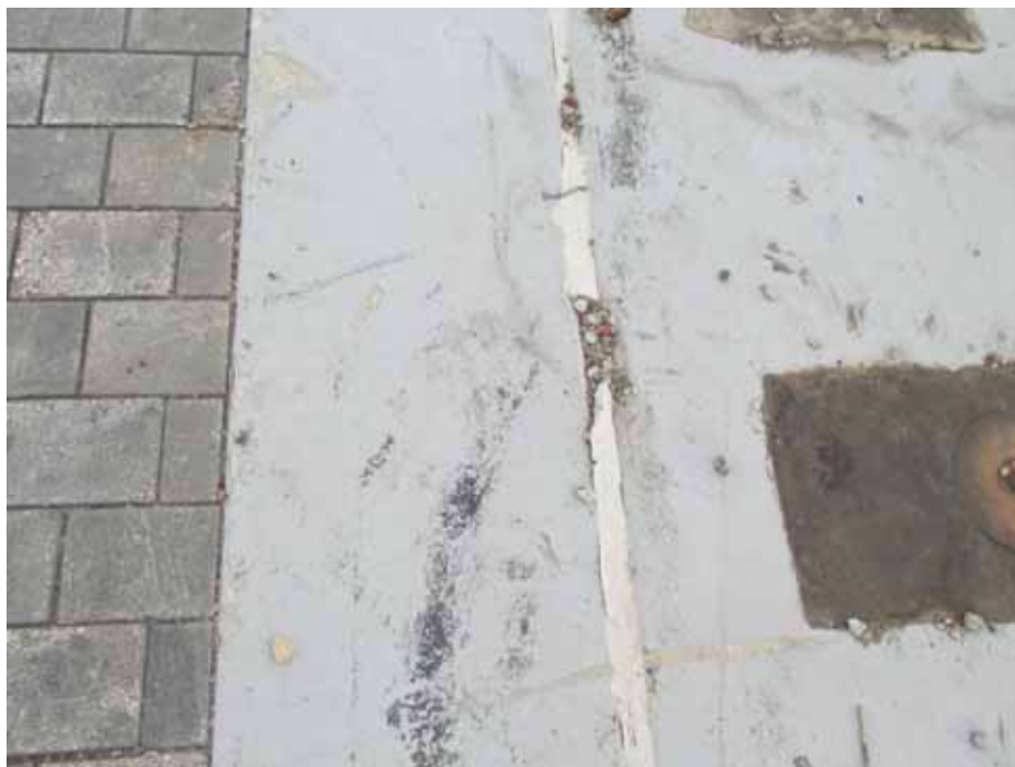
Photo 6: 11/5/13 – White caulk in seam (non-ACM).
