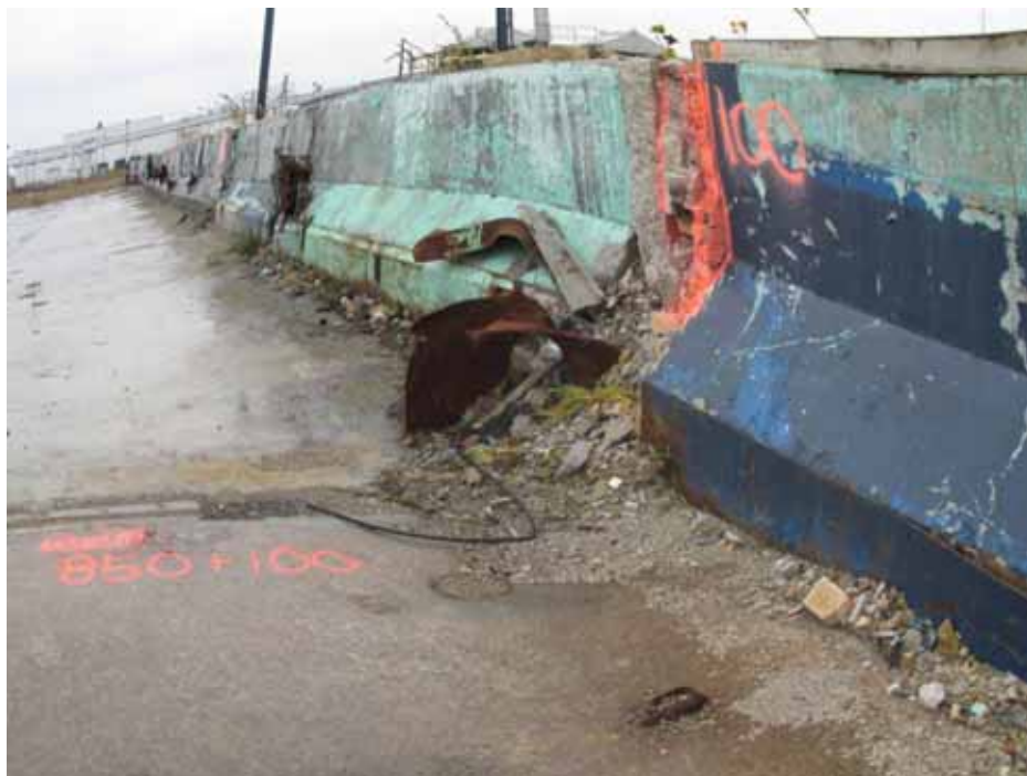
Photo 46: 11/11/13 – Grid Q2 with miscellaneous debris along wall.
