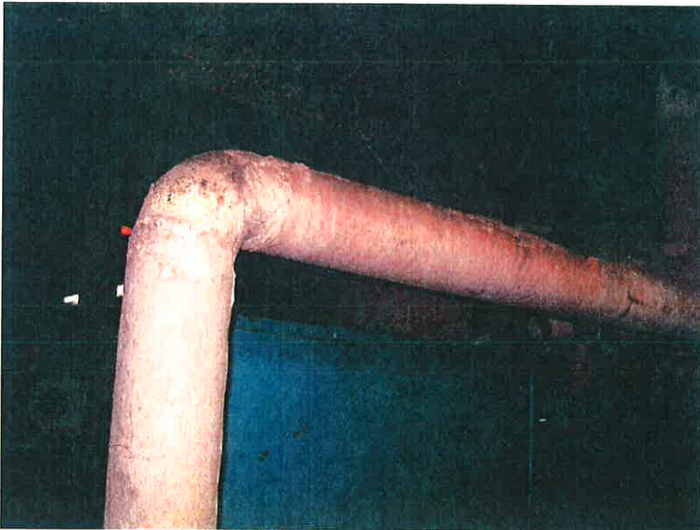
Continuation of labeled asbestos pipe insulation.
