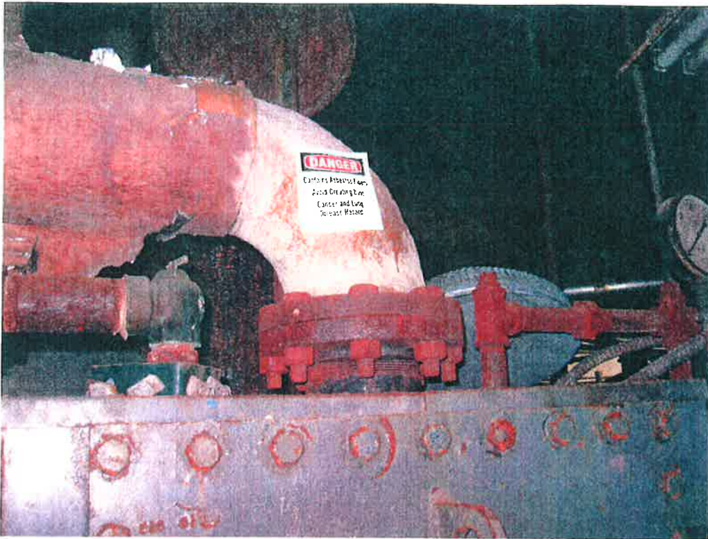
Labeled asbestos on boiler piping in basement of warehouse.
