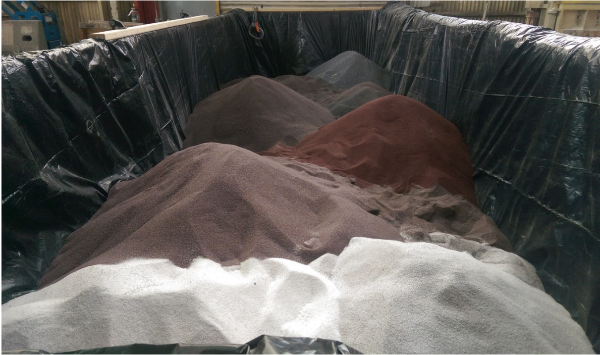
Photograph 37: View of different types of grit material found on-Site being consolidated for disposal.
