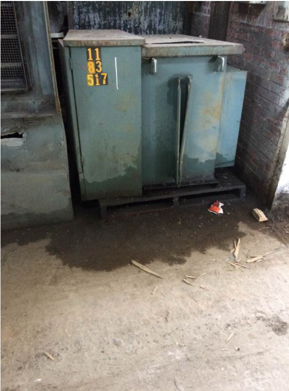
Photograph 6: View of transformer in Middle Room potentially containing transformer oil. Note spilled material of floor suspected to be transformer oil.
