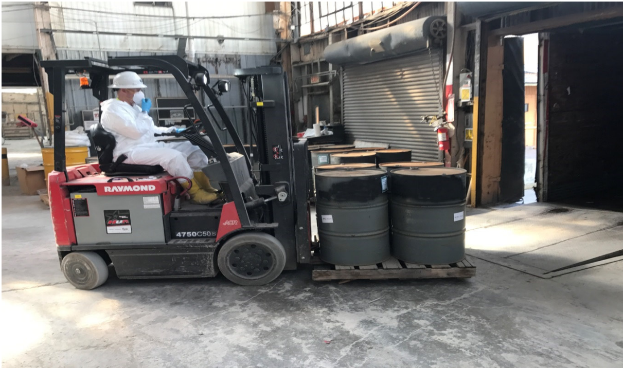
Photograph 29: View of material been loaded onto truck for transport to disposal facility.
