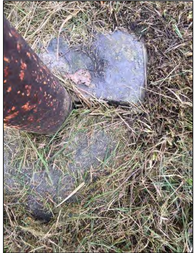
MW BR-1 broken pad, needs to be repaired
