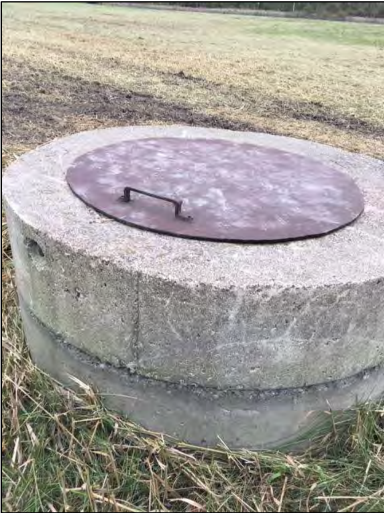
Sump Collection Tank (LS-1)
